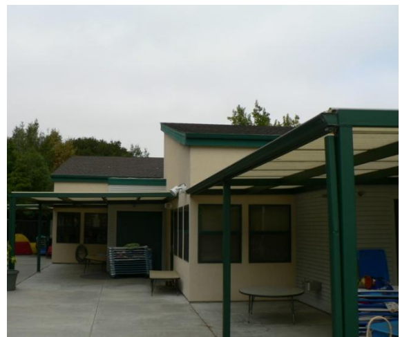
Figure 9 shows a view of Sections 1 and 2, which are on a shingle roof that is pitched at about 12°
