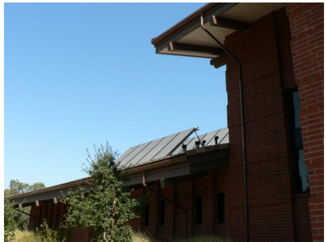
Figure 6 shows the existing solar thermal collectors
