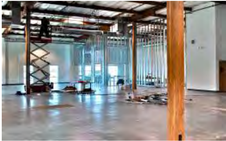
Tenant improvements underway at 3573 Haven Ave. to create smaller, collaborative R&D suites. For more information contact Greg DeLong at CBRE
