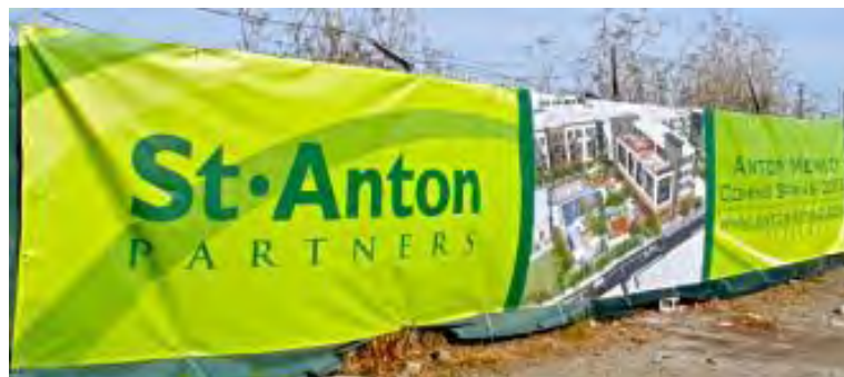
Construction underway at Anton Menlo, a 400 unit multi-family housing development geared towards Gen Y. The project includes collaborative spaces such as a pool, roof top deck, yoga room and iCafe. For more information read the Silicon Valley Business Journal's recent article on the project.
