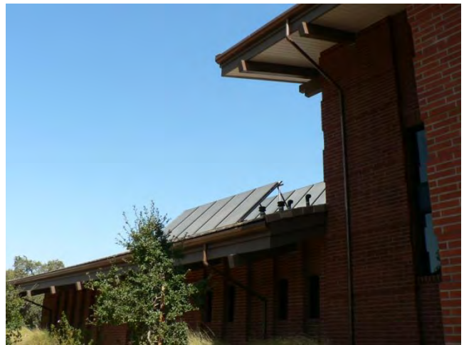
Figure 6 shows the existing solar thermal collectors
