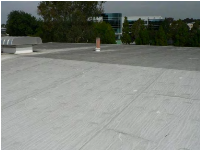
Figure 14 shows a view of Section 6, which is the highest area of the Community Center rooftop
