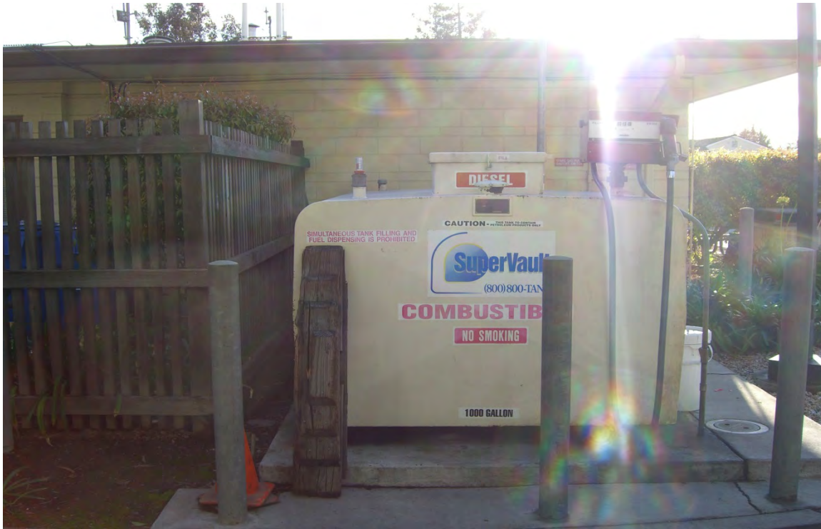
Fire Station No. 2: Looking west toward existing kitchen of Fire Station 2 and gas tank
