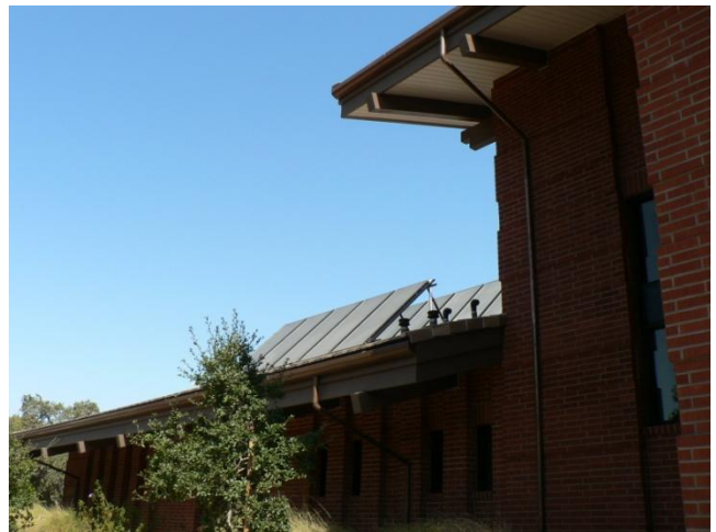
Figure 6 shows the existing solar thermal collectors
