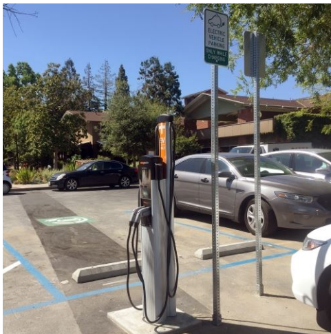
Electric vehicle charging at City Hall
