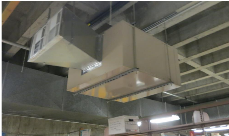
Basement Work Room Air Handler – No Outside Air Connection.
