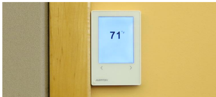
New "Alerton" Control Thermostat – Typical all Spaces
