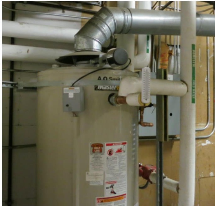
New Domestic Water Heater and Pump.
