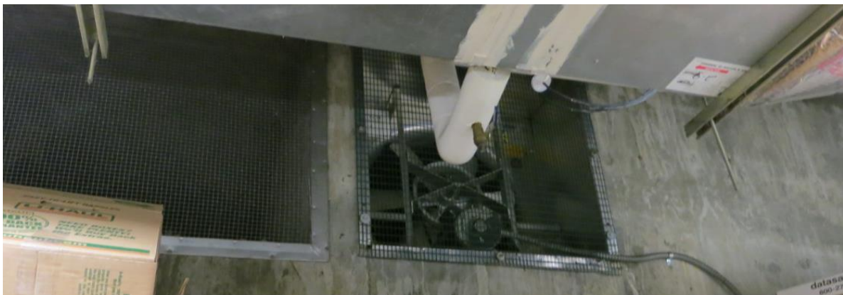
Basement – Abandoned Exhaust Fan. (served old cooling tower)
