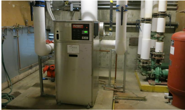
New Hydronic Heating Boiler
