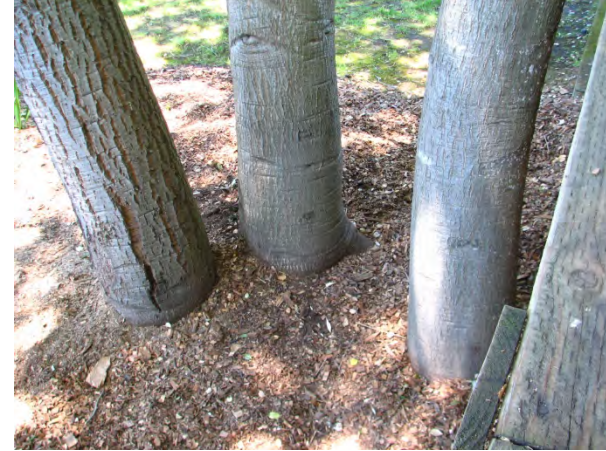
Coast live oak #7 has three mainstems (trunks) which are buried in fill soil, and require hand-excitation (this is a neighbor tree).
