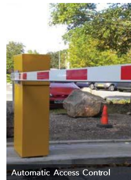
Automatic Access Control
