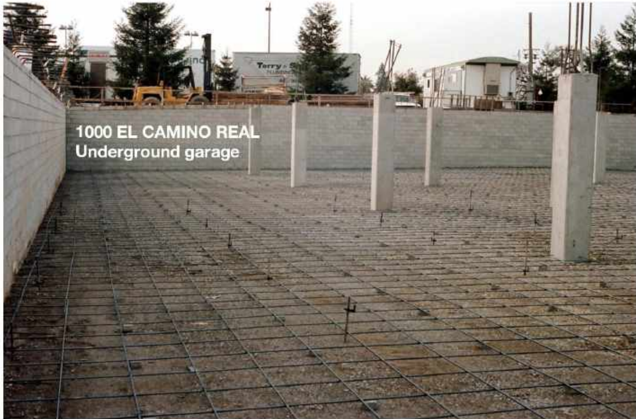
A-1.3 - Construction of underground garage at 1000 El Camino Real in the 1980s.
