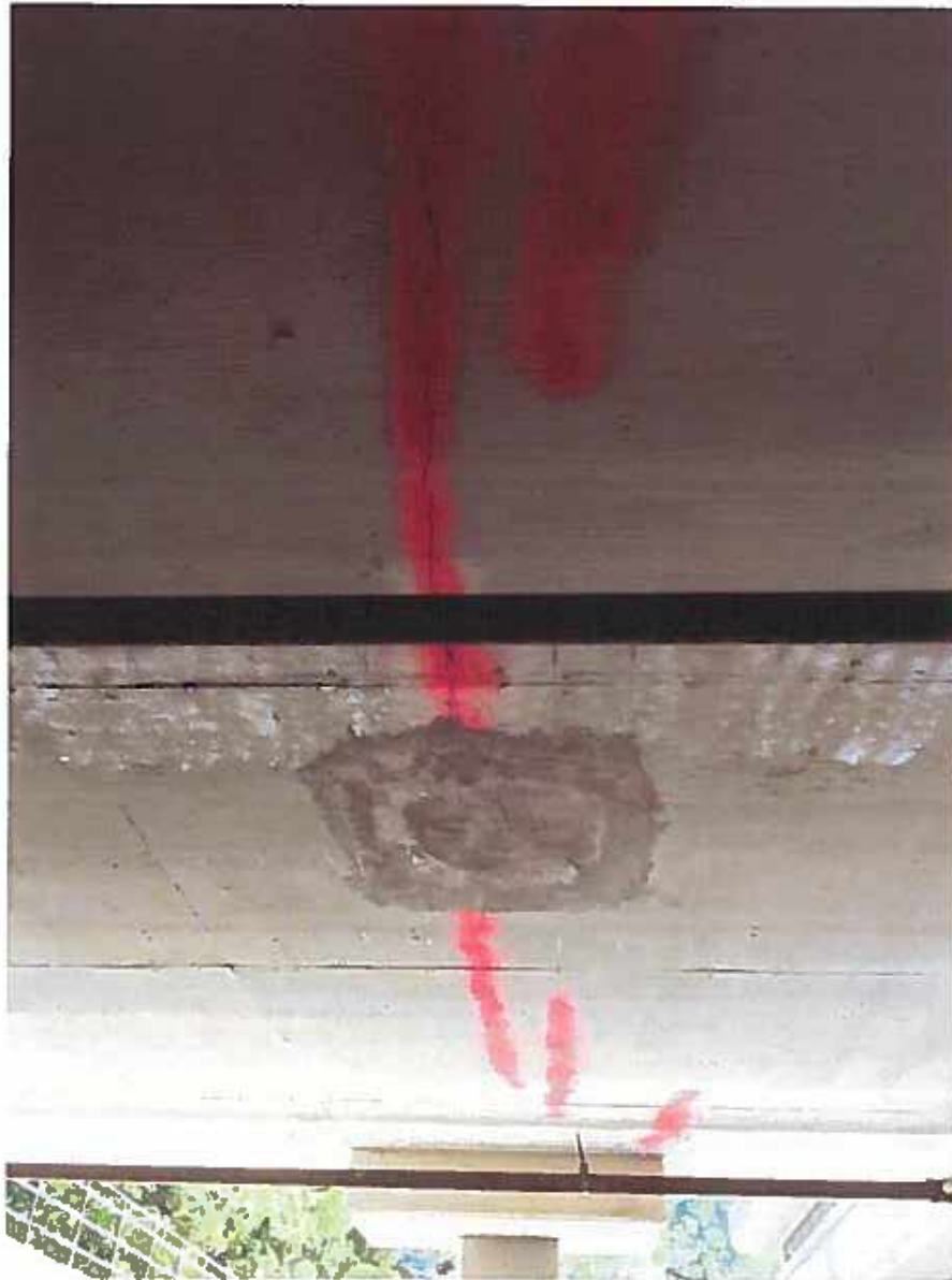
Photo 2 – Podium slab cracks along with chip and patch regions at gridline 2
