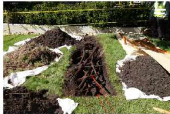
THICK TANGLE OF TREE ROOTS OVER THE PODIUM AND UNDERGROUND GARAGE PODIUM SLAB WATERPROOFING
