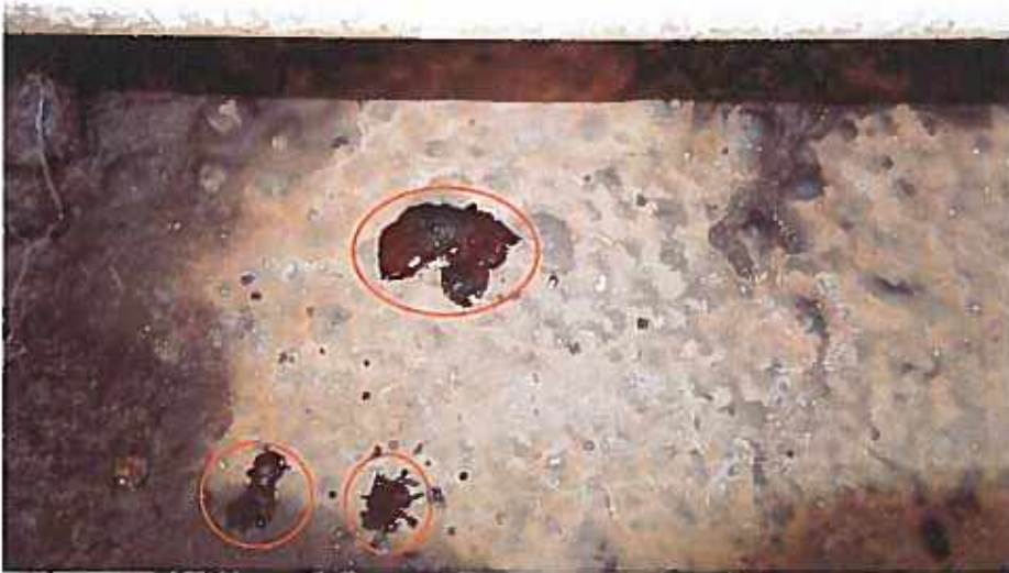
Figure 16 Sliced blisters seeping trapped water that was below the waterproofing – indicating that moisture is moving through the waterproofing membrane.
