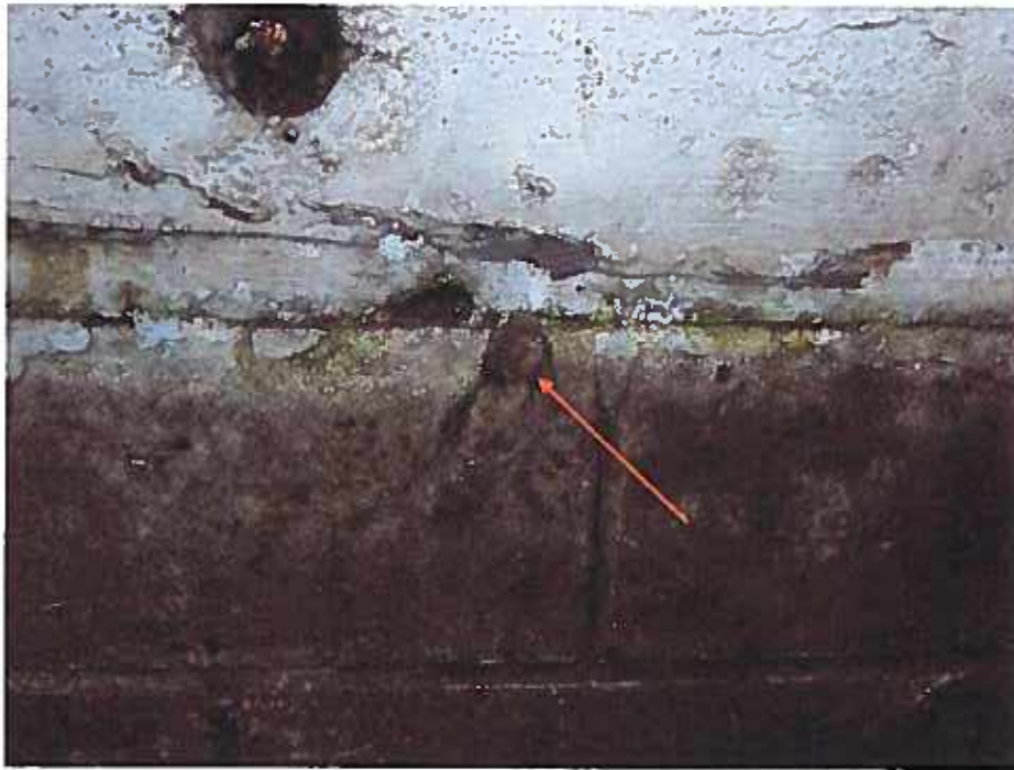
Figure 24 Close-up of attachment pin. Attachment frequency was insufficient.
