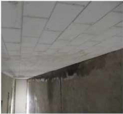
DAMAGE TO PODIUM WATER-PROOFING AT LOCATIONS ADJACENT TO REDWOOD TREE PLANTING.
