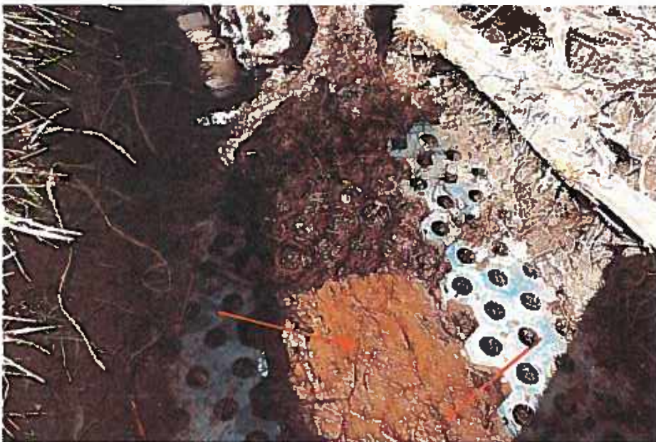
Figure 9 Destructive testing (DT) area where grass, soil, etc. to expose waterproofing. Note how the small root hairs are embedded within the waterproofing membrane.
