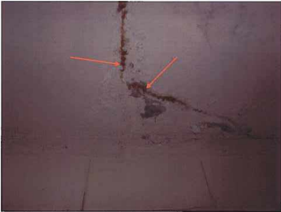
Figure 6 Active dripping from underside of podium slab.
