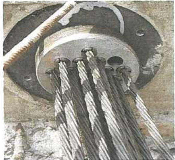
Post-tensioned tendon anchorage. Four-piece "lock-off" wedges are visible holding each strand
