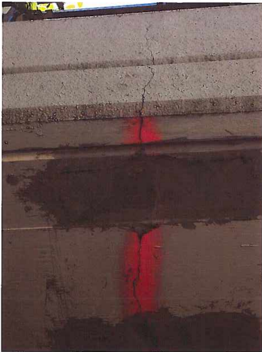
Photo 1 – Podium slab cracks along with chip and patch regions at gridlines 2.5/H1
