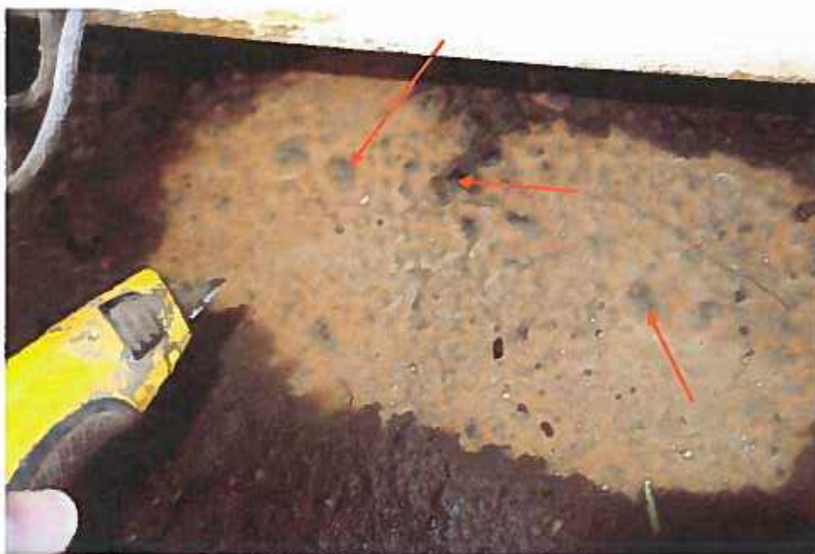
Figure 15 Close-up of waterproofing membrane showing blistering.
