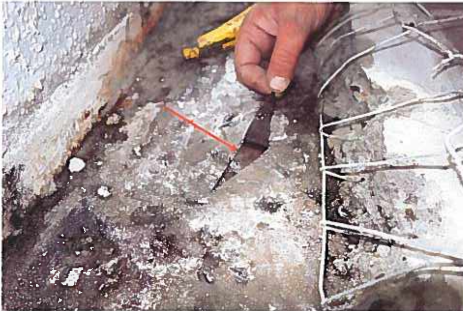
Figure 20 Adhesion pull-test was performed on the waterproofing membrane. Adhesion was poor.
