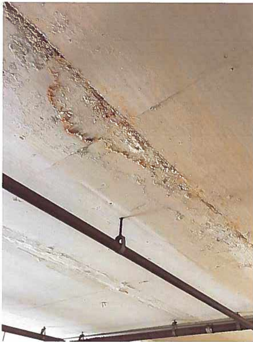
Photo 7 - Concrete discoloring at the closure strip near gridline 6.8/B.5
