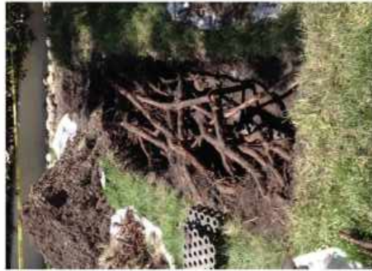
EXPOSED ROOTS OF REDWOODS INTRUDING ON PODIUM INTEGRITY
