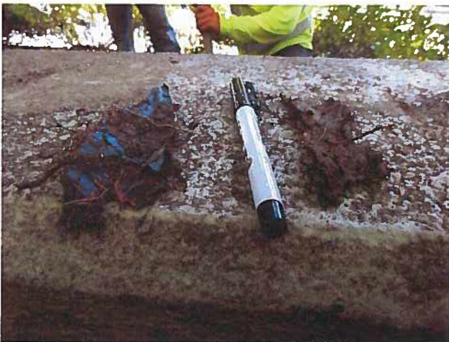
Figure 25 Samples of self-adhering membrane taken from location. Note the extent of root damage caused by the roots penetrating the membrane.
