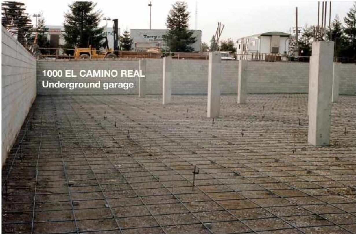
A-1.3 - Construction of underground garage at 1000 El Camino Real in the 1980s. The post-tensioned slab in question sits on top of these walls and pillars.
