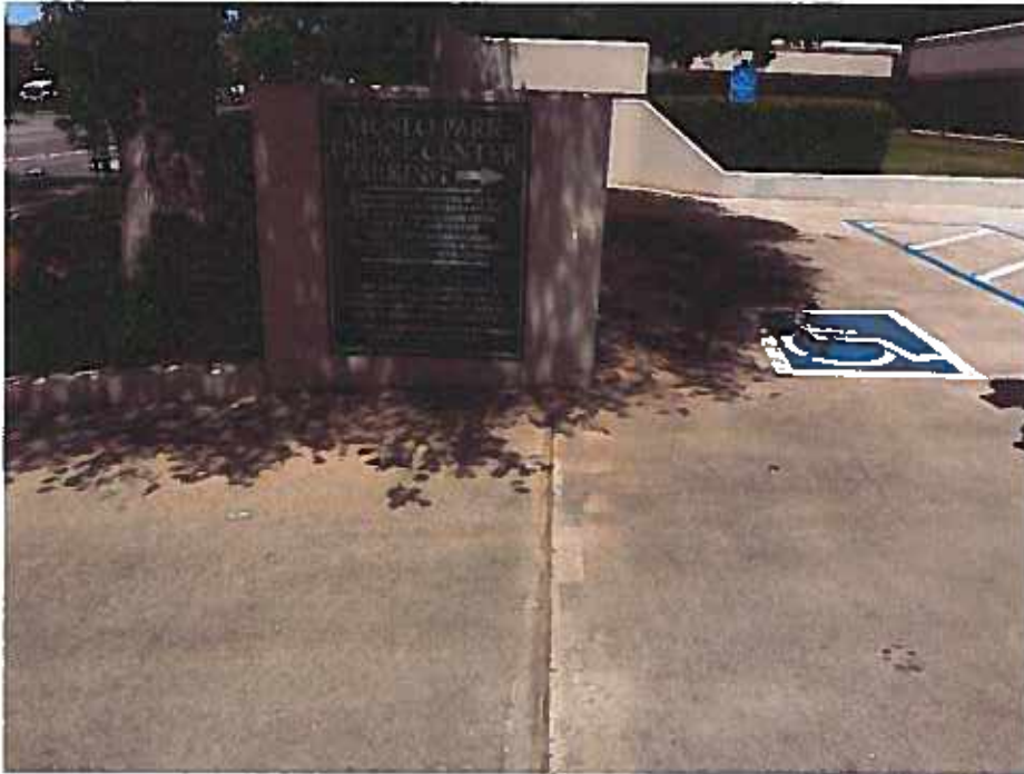
Figure 28 Topcoat of existing parking deck is aged and maintenance is recommended.
