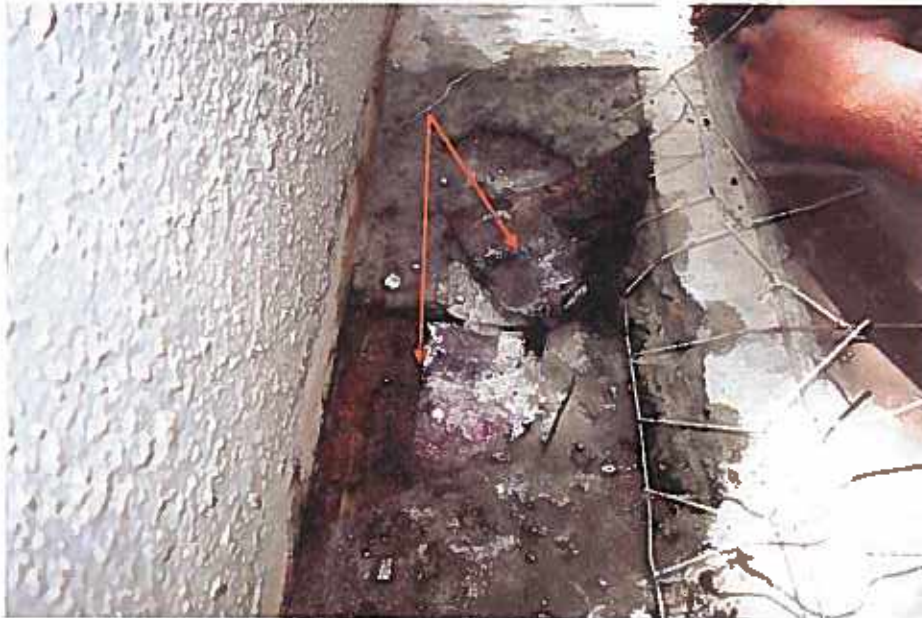
Figure 22 Note moisture below membrane, indicating water intrusion is occurring. Water below the waterproofing membrane can travel through voids and unadhered portions of the membrane.
