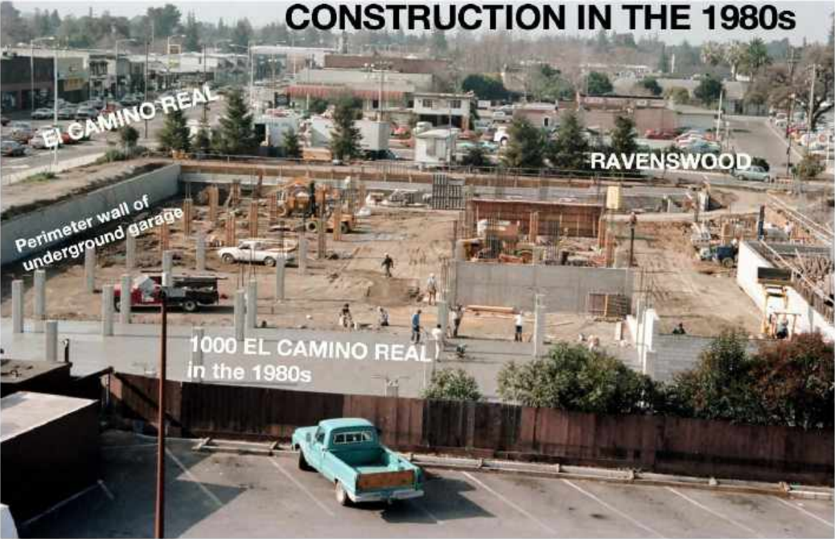
A-1.1 - Construction on the 1000 El Camino Real property in the 1980s. Note that the excavation for the underground garage covers almost the entire site.
