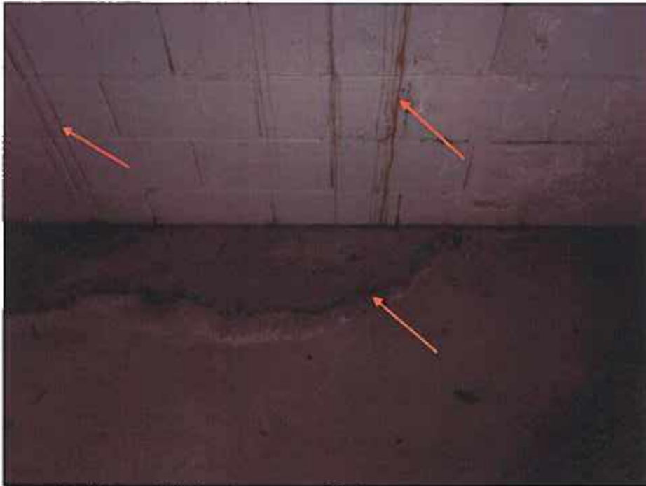
Figure 2 Staining on CMU foundation walls; staining on floor; from water intrusion.
