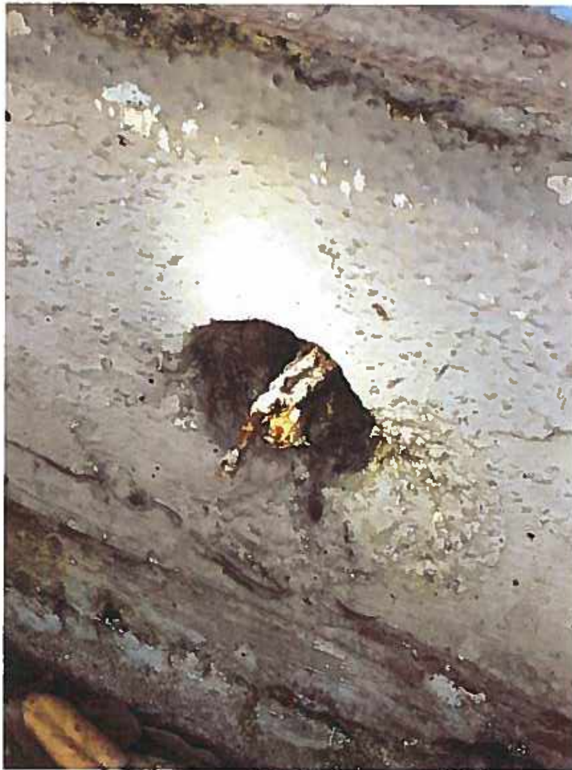
Photo 6 - Exposed P/T tendon showing signs of corrosion
