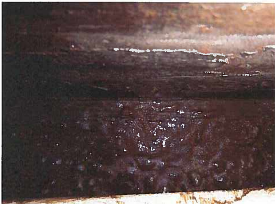
Figure 18 Note the network of blisters within the waterproofing membrane.
