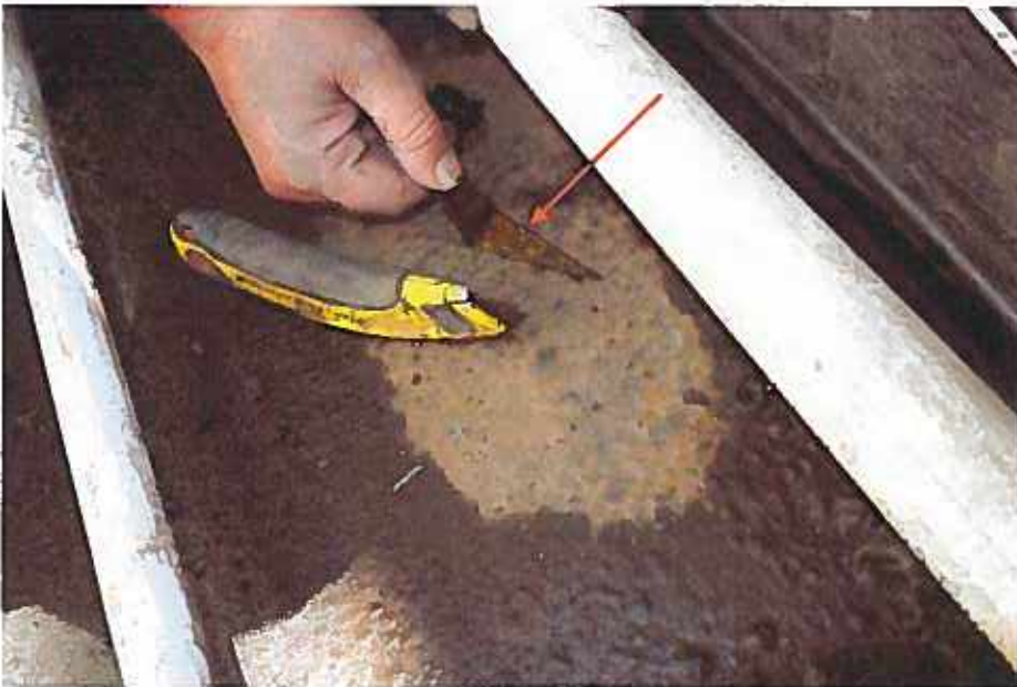
Figure 17 Adhesion pull test was performed on the waterproofing membrane. Adhesion was poor.
