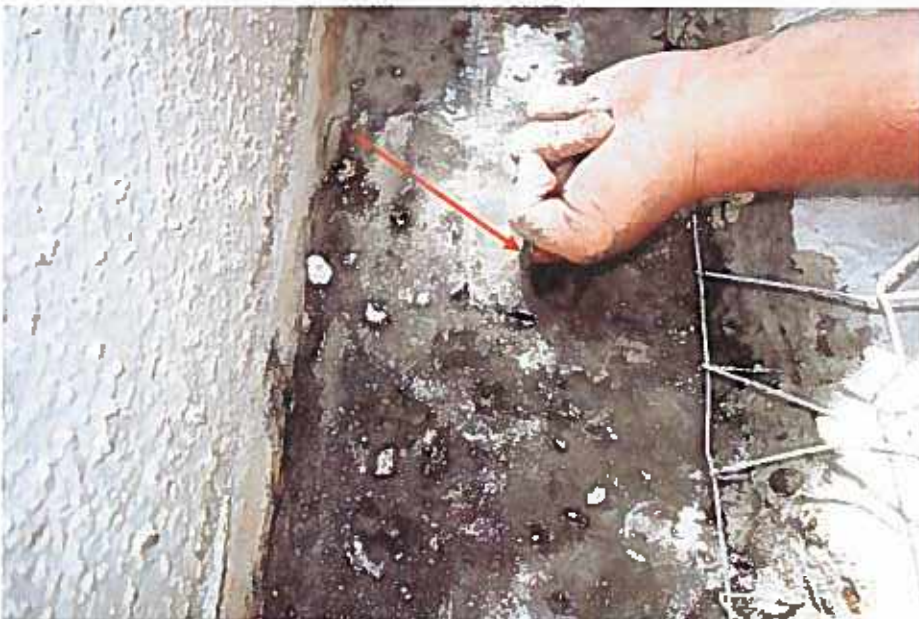
Figure 21 Note the void in the membrane where it is unadhered to the slab below.
