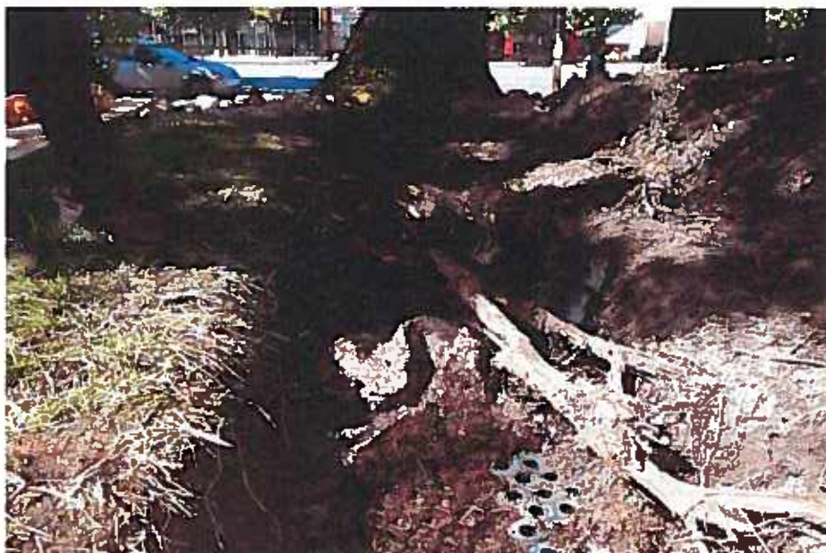
Figure 10 DT location showing large root system extending throughout the podium area. Root system is damaging the waterproofing membrane through surface abrasion and by penetrating the membrane - opening pathways for water intrusion into the podium slab.
