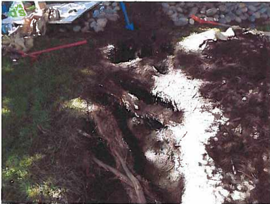
Figure 12 Large roots extending from trees along El Camino Real toward the building (above the podium area.) These roots are throughout the podium.
