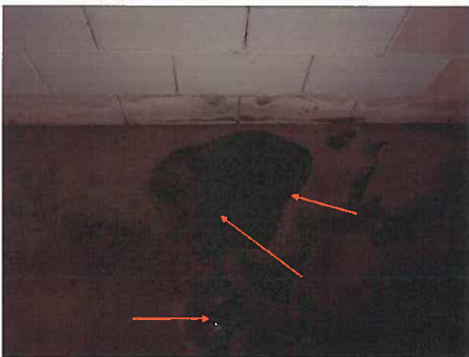
Figure 5 Water with rust staining from podium slab leak above.
