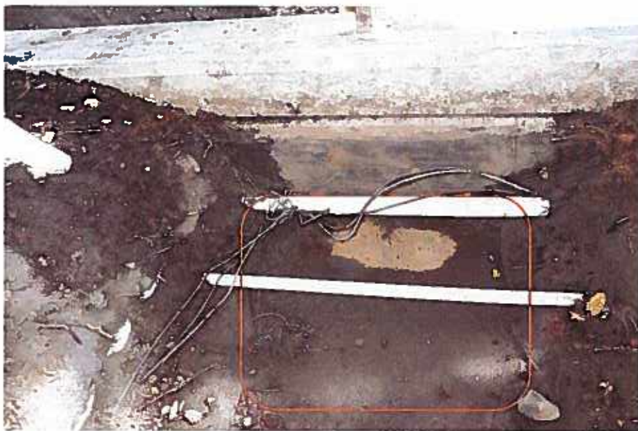
Figure 14 DT location in courtyard planter - exposing waterproofing membrane.
