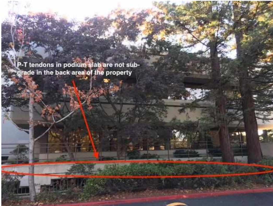
A-1.9 – View on the north side of the 1000 El Camino Real building showing that the Post tension (P-T) tendons are above grade, which is a different condition than in the front.
