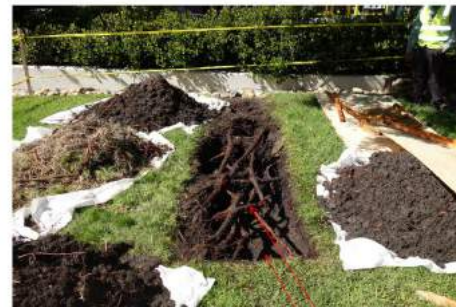
THICK TANGLE OF TREE ROOTS OVER THE PODIUM AND UNDERGROUND GARAGE PODIUM SLAB WATERPROOFING
