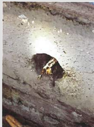
Photo 6 - Exposed P/T tendon showing signs of corrosion
