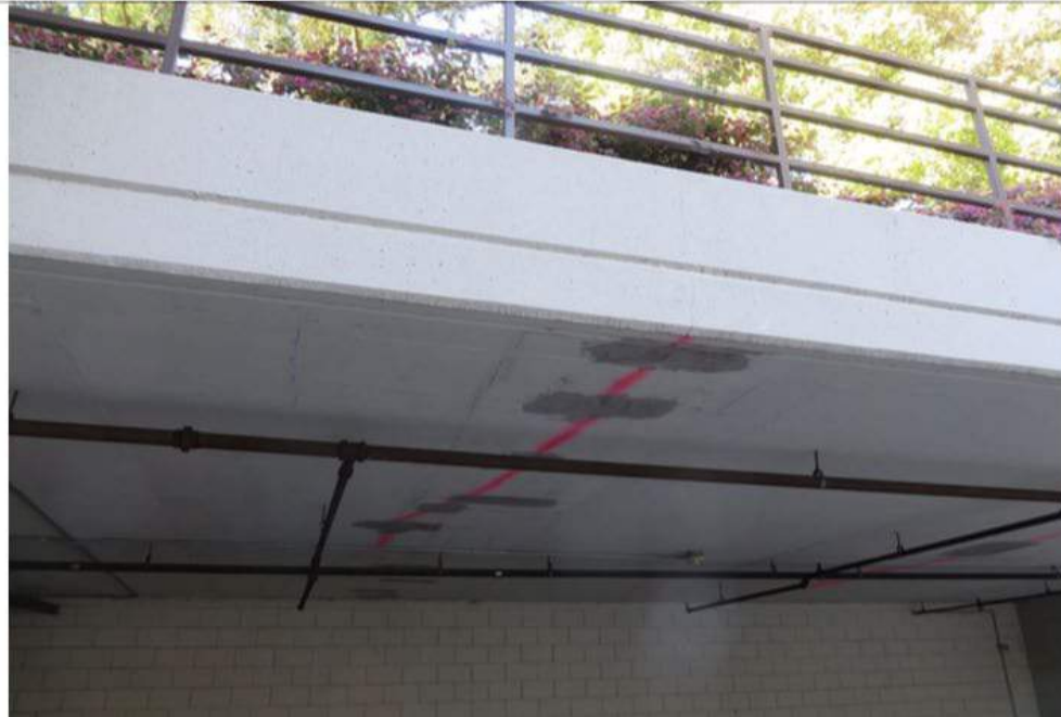
POST-TENSIONED CABLES BROKEN
