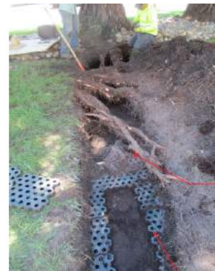
THICK TANGLE OF TREE ROOTS OVER THE PODIUM AND UNDERGROUND GARAGE
