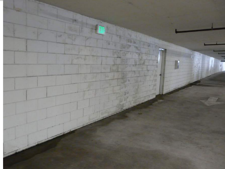
WATER INTRUSION AND DAMAGE TO UNDERGROUND GARAGE WALL
