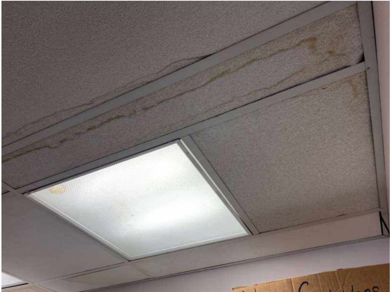
MENLO PARK PUBLIC LIBRARY Interior water damage due to roof leaks. Photo taken at Menlo Park Main Library on March 21, 2022
