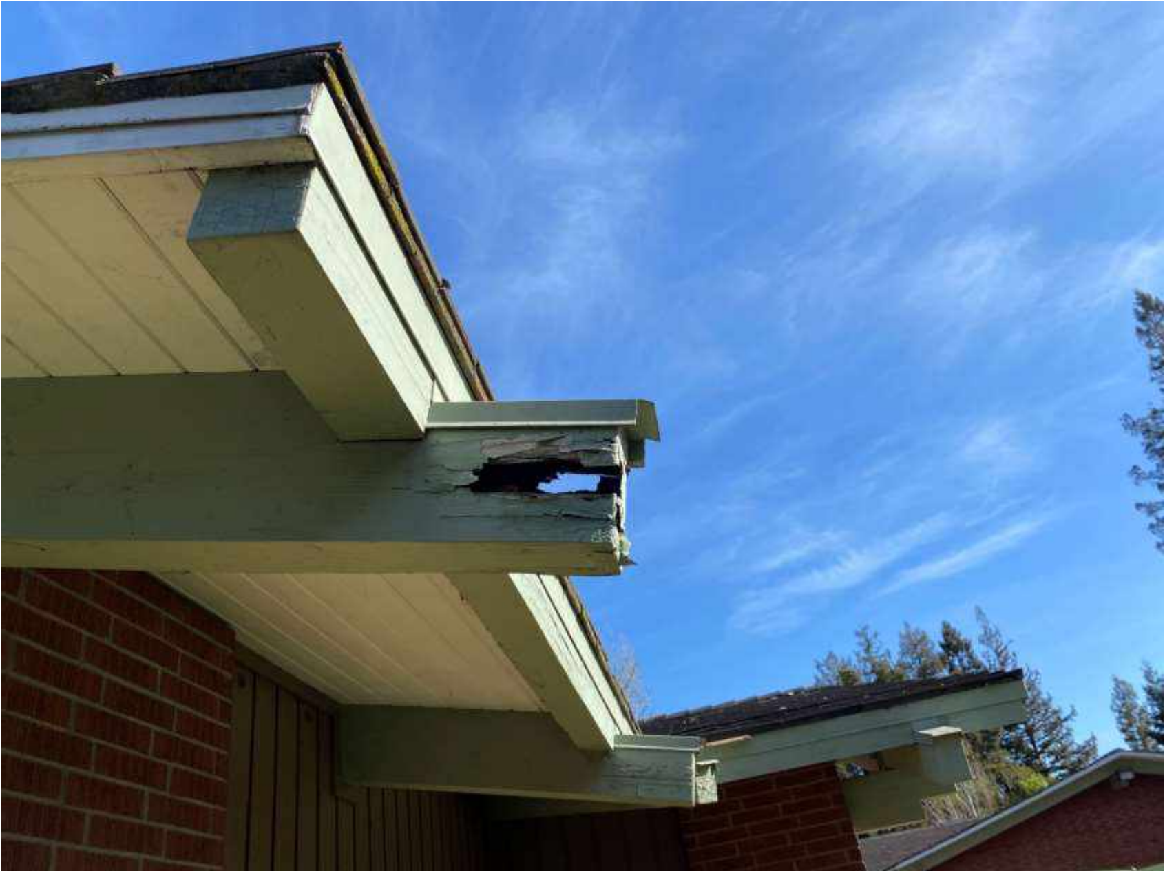
MENLO PARK PUBLIC LIBRARY Damaged/failing roof support beam. Photo taken at Menlo Park Main Library on March 21, 2022
