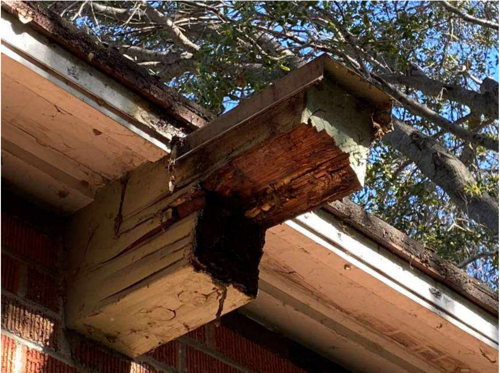
MENLO PARK PUBLIC LIBRARY Damaged/failing roof support beam. Photo taken at Menlo Park Main Library on March 21, 2022
