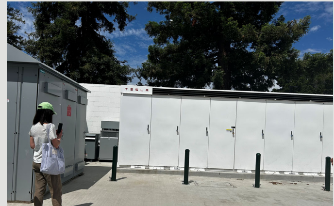
Battery storage at the Belle Haven Community Campus
