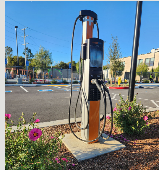
Level 2 EV charger at Belle Haven Community Campus
