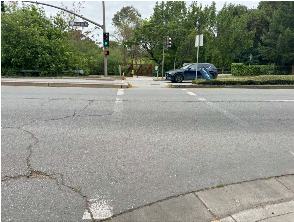
Figure 5-27 Worn out crosswalk striping
