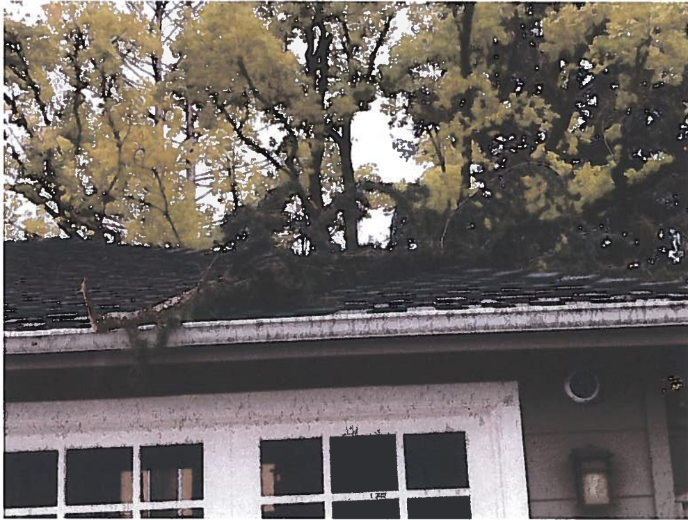
Photo 2: Recent fallen limb on house
