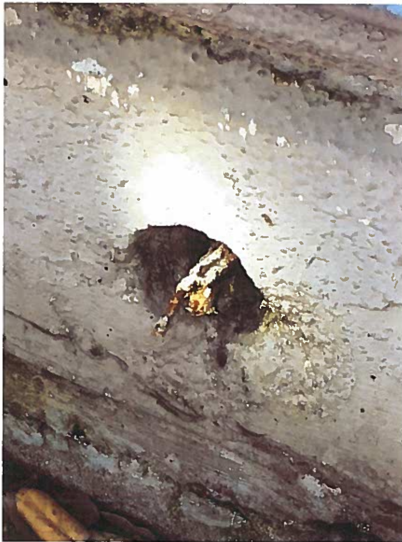
Photo 6 - Exposed P/T tendon showing signs of corrosion
