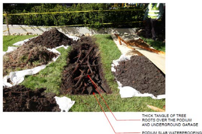
Figure 2: Additional Root Exposure
