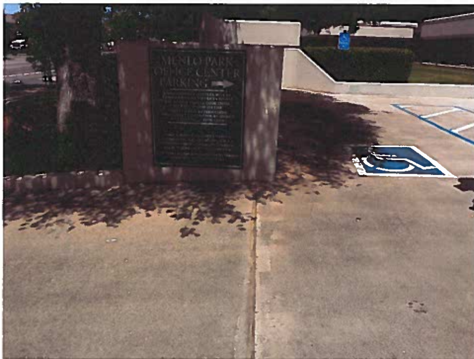
Figure 26 Topcoat of existing parking deck is aged and maintenance is recommended.
