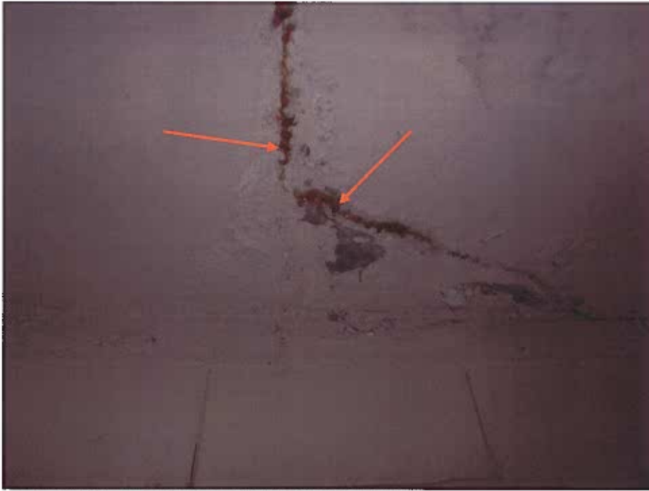
Figure 6 Active dripping from underside of podium slab.
