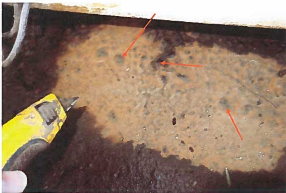
Figure 15 Close-up of waterproofing membrane showing blistering.
