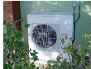
Heat pump condenser evaporator unit
