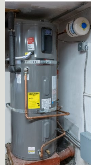
Installed heat pump water heater
