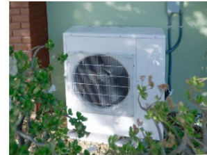
Heat pump condenser evaporator unit
