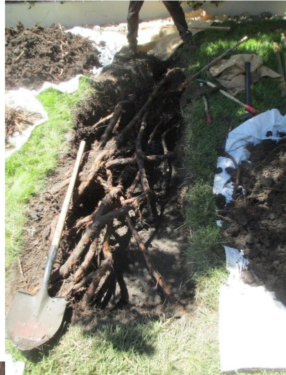
Photo 3. Photo to the right shows the massive amount of roots found in the turf area. All of these roots would need to be removed to accommodate the waterproofing.
