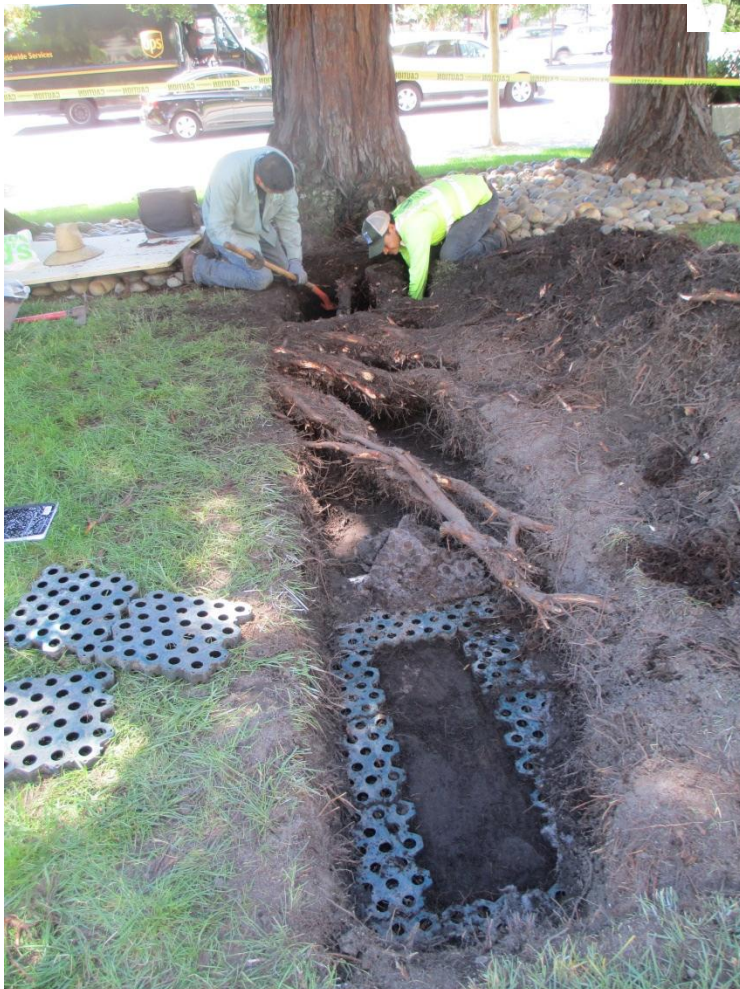
Photo 4. Photo to the left shows the old water proofing and protection open for inspection. Significant root cutting was needed to gain access to the surface of the garage roof. People doing the excavation are working at the edge of the outer wall of the below ground garage. Cutting large roots so close to the tree will compromise the root anchoring and tree stability. Most likely "target" would be El Camino Real in the background.
