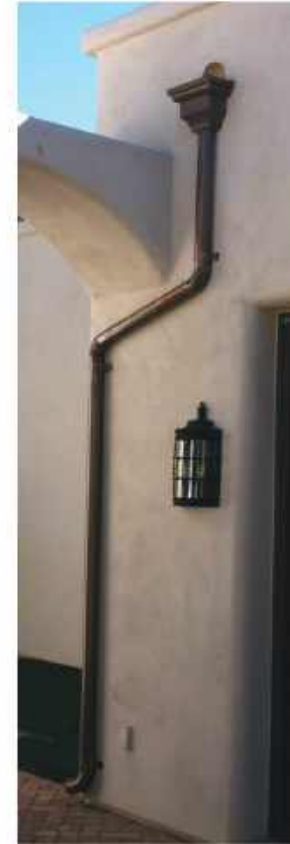
RAIN WATER SCUPPER AND LEADER
