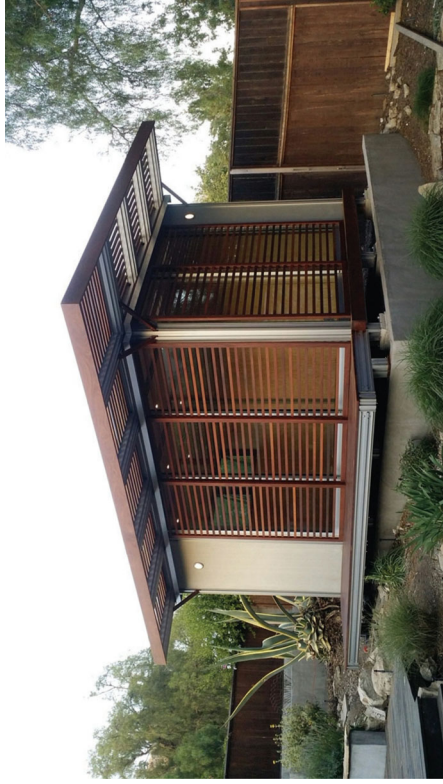
kiHAUS k4.10.8 at a Neutra house in Palos Verdes CA with smooth cement board finish to match existing smooth trowel stucco finish
