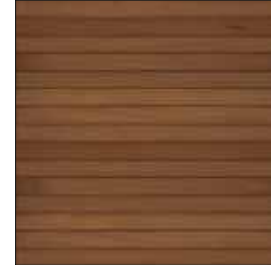
stained wood balcony soffits
