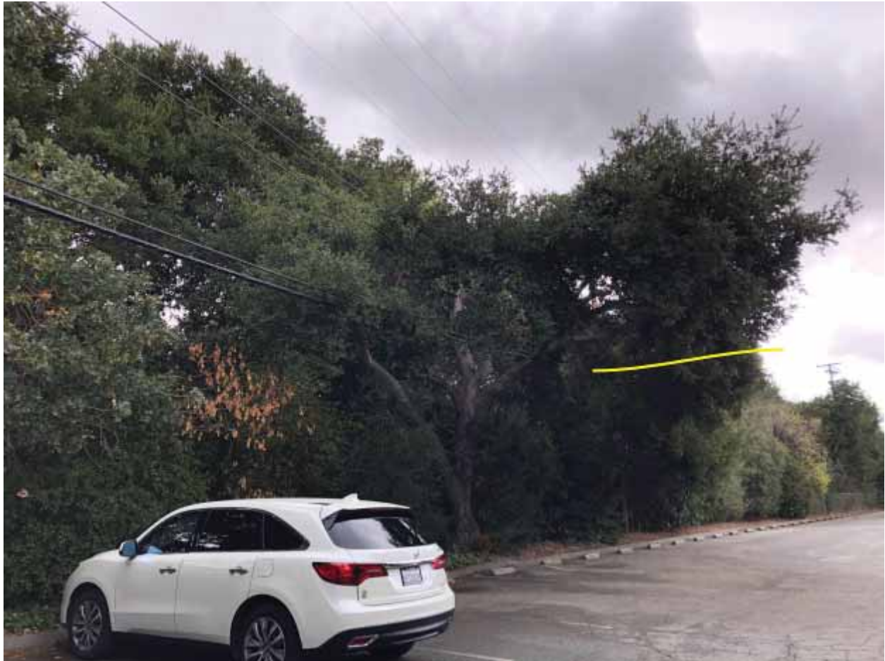
Image 13: approximate clearance pruning needed for trees #1650 (left, pruned for line clearance) and 1651 (right, extreme lean over parking; canopies touching)
