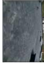
FLAT ROOF WITH TPO ROOFING WITH BLUE FINISH MANUFACTURER - GAF OR EG
