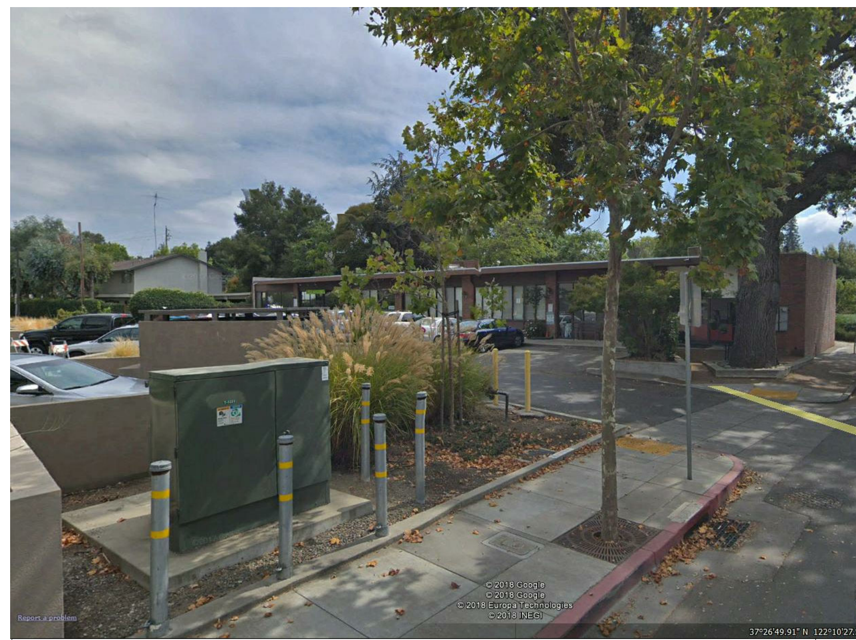
PG&E PAD MOUNTED TRANSFORMER ACROSS CAMBRIDGE FROM 201 EL CAMINO 4.
