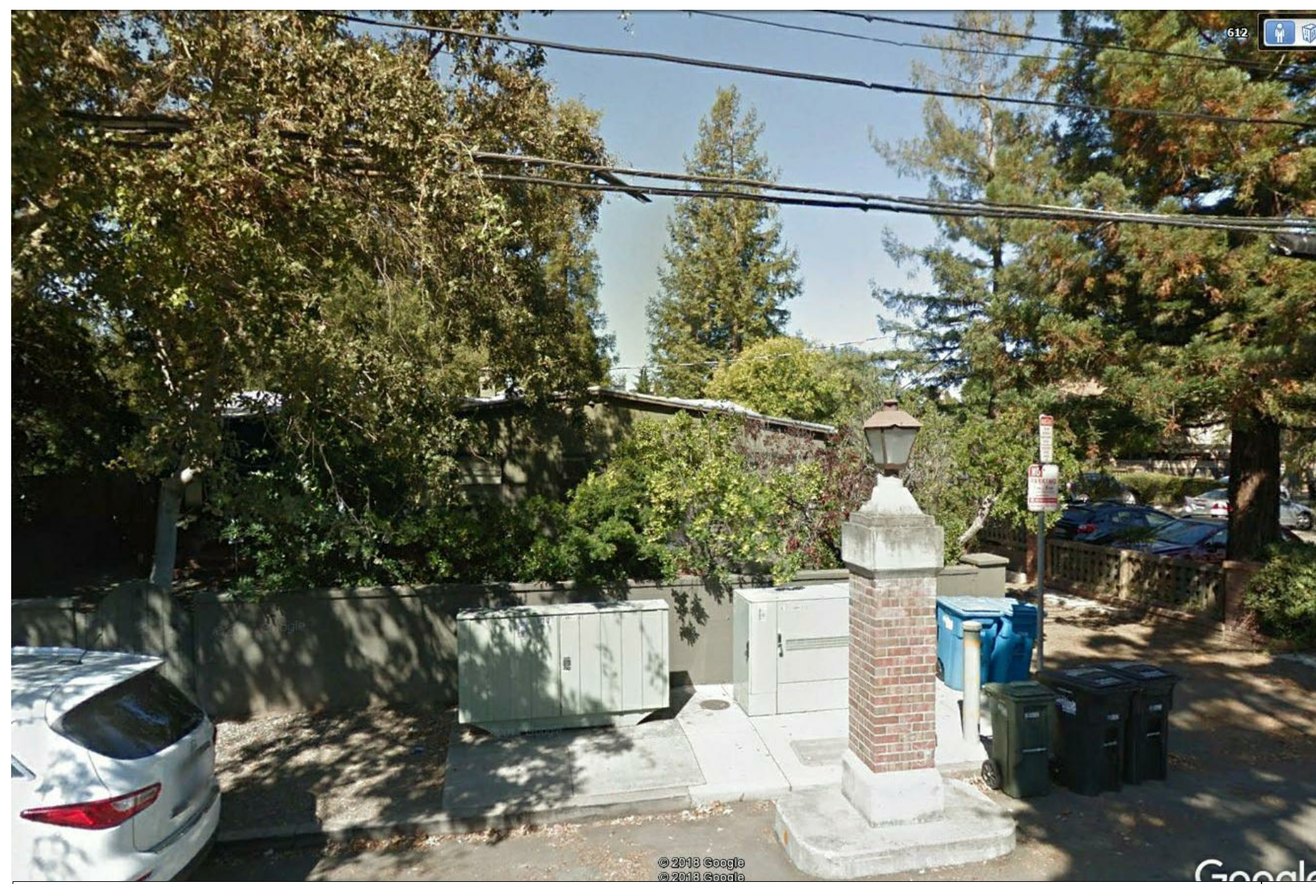
AT&T AND CABLES AT CAMBRIDGE 7.
