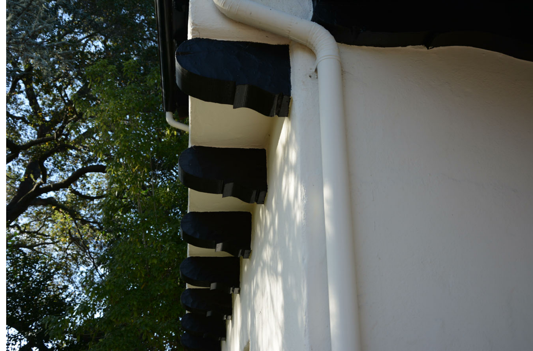
CORBELS UNDER SECOND FLOOR OVERHANG 9.
