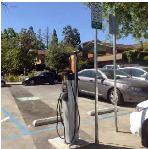
Electric vehicle charging at City Hall
