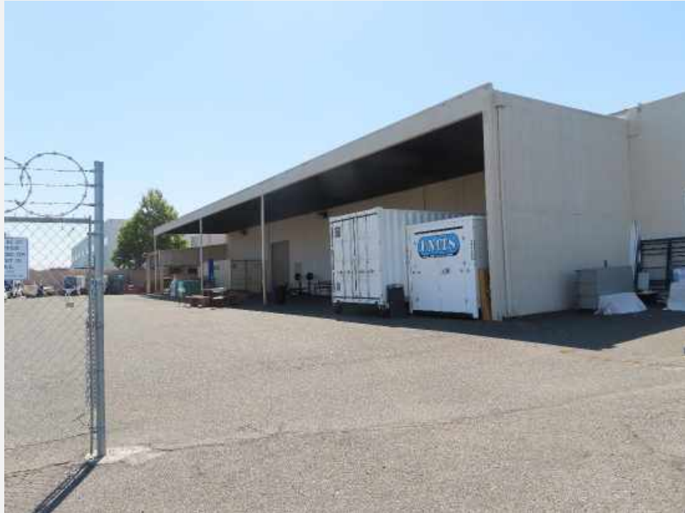
Exhibit 4. Shelters attached to the rear (north) elevation of the building, view looking southeast (IMG_0855).
