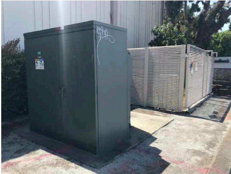
Photograph 15: Transformer and emergency generator at the Site.
