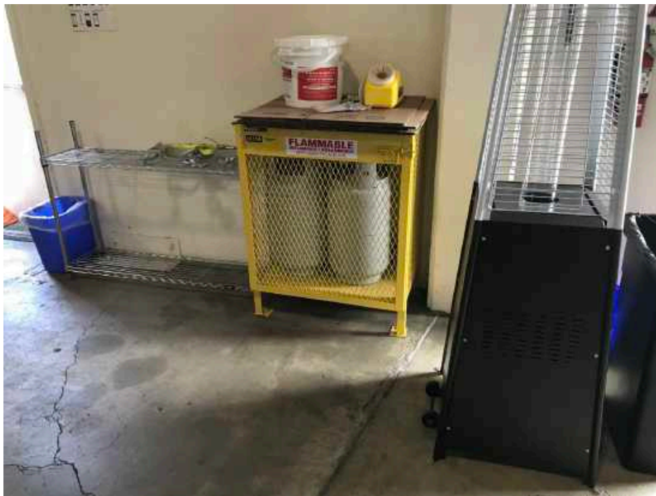
Photograph 4: Propane tank storage in building at 985 O'Brien Drive.
