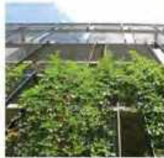
E1 GREEN SCREEN STEEL FRAMED PANEL WITH STEEL WIRE GRIDS 24X 4' WIDE PANELS SPACED WITH 4" GAPS HORIZONTALLY
