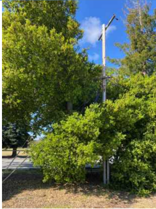
PHOTO 13: View of overhead power pole in the southwest portion of the Site, looking southwest.
