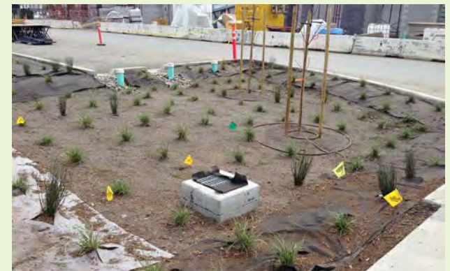
▲ The clean outs for this project could have been better placed and not sited immediately downstream of the curb cut inlets.
