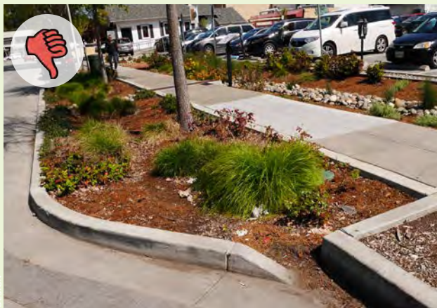
▲ This green street unfortunately uses organic mulch in the flow path of water which will in time float away.
