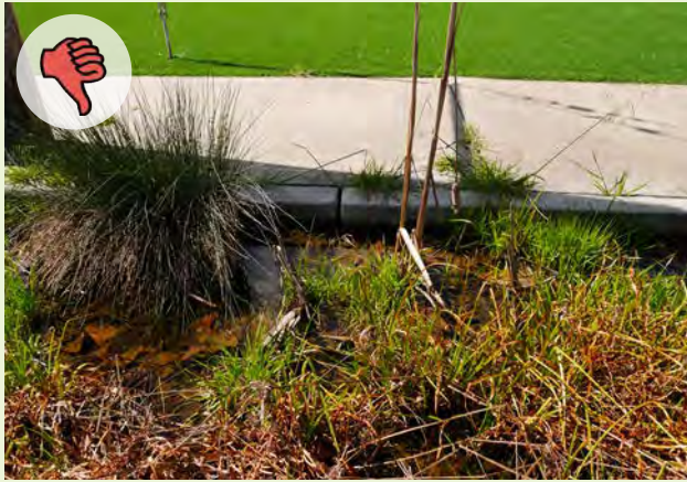
▲ This stormwater curb extension suffers from poor infiltration to the point where standing water occurs frequently enough to allow for algae growth and invasive plant species to take over the landscape.
