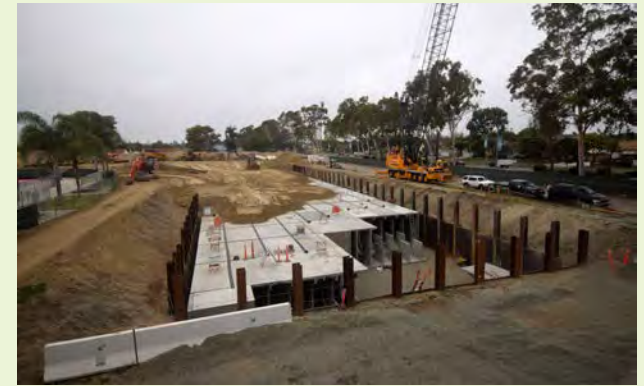
▲ Treated water is piped approximately 650 feet from the channel and treatment equipment to the underground facilities so that the underground facilities can be placed under the park’s open ballfields.
