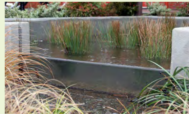
▲ This adjustable weir can control how much water is to be retained within a rain garden.
