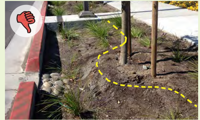
▲ The yellow dashed line shows how the grading within this stormwater curb extension is warped due to the tree placed above and outside the wetted zone. This scenario reduces the retention capacity of the landscape.
