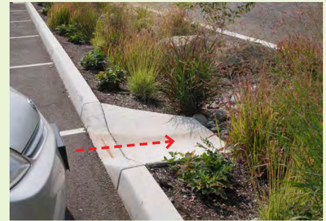
▲ A standard curb with wings allows stormwater runoff to enter a stormwater facility. The wings help retain the side slope grade on each side of the curb cut opening.
