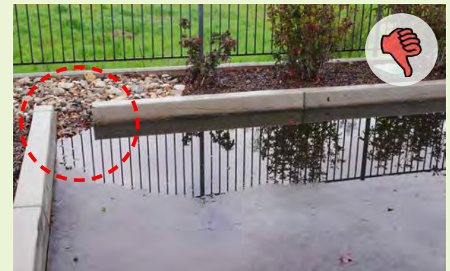
▲ A curb cut blocked by cobbles and sediment prevents water flow into this stormwater facility. There is not enough grade change between the curb cut entry and the finish grade of landscaping.
