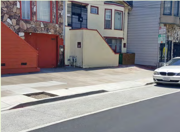
▲ Pervious concrete used in parking lane in a highly constrained urban area.
