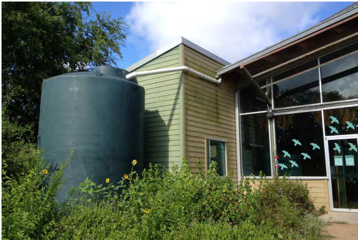
▲ EXAMPLE: This 5,000-gallon rainwater harvesting system at the education building of the World Birding Center in Edinburg provides irrigation for nearby flowering plants and shrubs.
