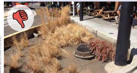
Poor, Overhaul Maintenance Routine
