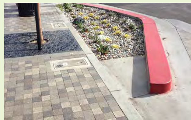
▲ While this is a good concrete pad, the elevation needs to be lowered at least 2 inches to allow for sediment capture.
