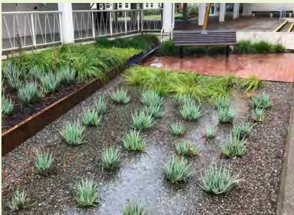
▲ This rain garden is graded very shallow to allow ponding of water, but it is not excessively deep or have steep side slopes. Ultimately this rain garden will perform better over time and will be easier to maintain.
