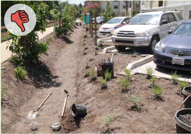
▲ This newly installed green infrastructure facility will have consistent problems with erosion control and plant health issues because of steep side slope conditions (steeper than 3:1 slope).
