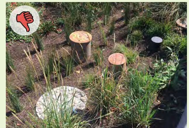
▲ Stormwater facility cleanouts and other utilities should be placed to be easily accessed and maintained, and not in the middle of the facility.
