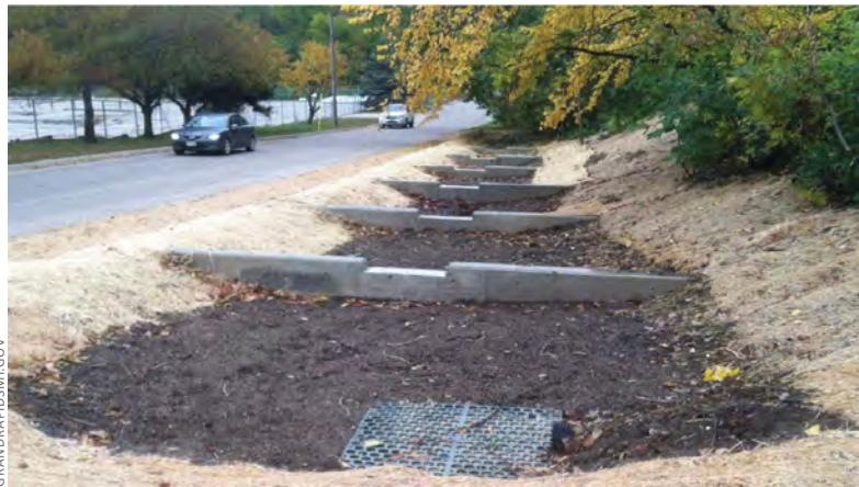
▲ This example uses stormwater planters instead of vegetated swales to gain treatment credits. The planters step down a gradual slope with check dams and are installed along the shoulder of a road, maintaining the rural character of the area.
