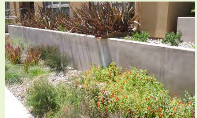
▲ This flat planter-style landscape is completely mulched with small rock to control erosion with water flow.
