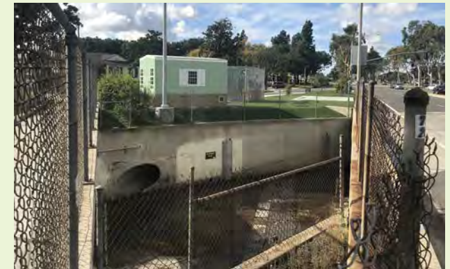
▲ The treatment and smart system equipment is located on a remnant parcel fronted by streets on three sides and the channel and a pedestrian bridge on the other. Some equipment is sited above ground, while other equipment is underground below the astroturf and concrete pad. Bolivar Park is in the background, center to left.
