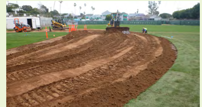
▲ Following the installation of underground infrastructure, the field is covered and restored. The captured and treated runoff is used to irrigate and to flush toilets at the park.
