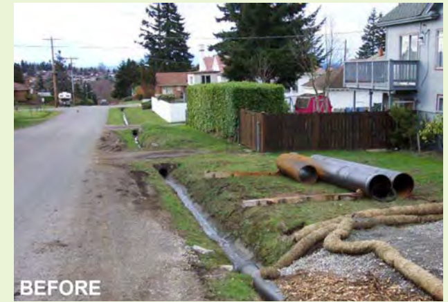
▲ BEFORE: An unimproved semi-rural road with ditches was selected to be retrofitted with green infrastructure facilities.
