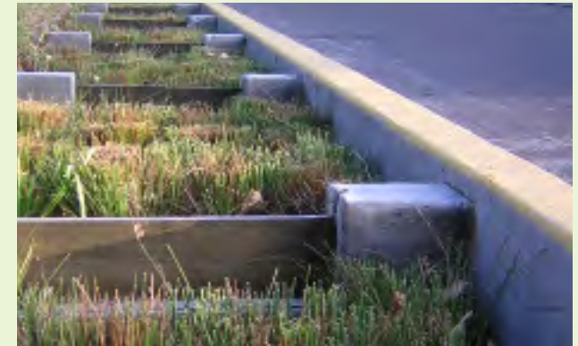
▲ Adjustable weirs within these stormwater planters allow for the flexibility of how much water is retained. These weirs are set to retain a maximum of 6 inches of water but can be lowered to retain less water if desired.
