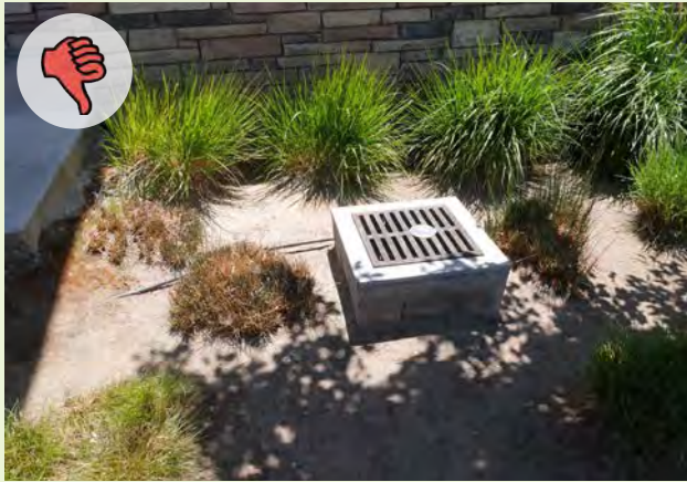
▲ This storm inlet's rim is placed at a fixed height of over 8 inches. If this rain garden does not infiltrate at a reasonable rate, it could suffer the effects of too much prolonged standing water.
