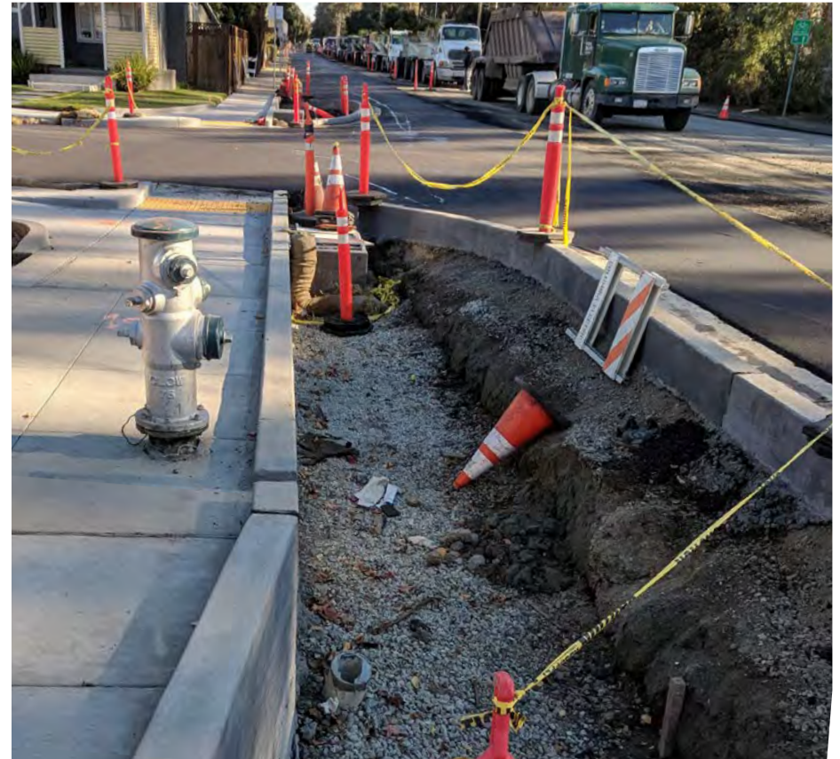
▲ Construction administration is important to ensure that the project is built according to the plans.
