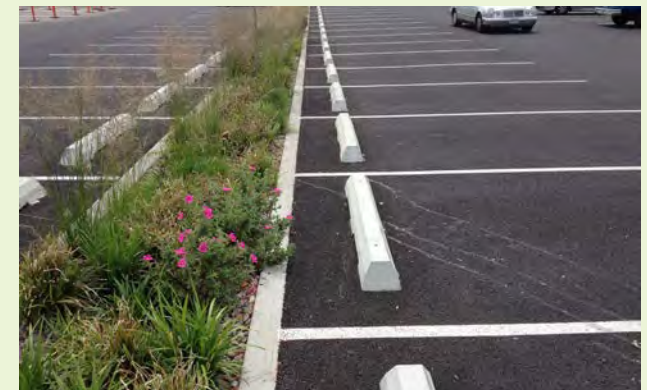
▲ An at-grade stormwater planter within the interior median of a parking lot.
