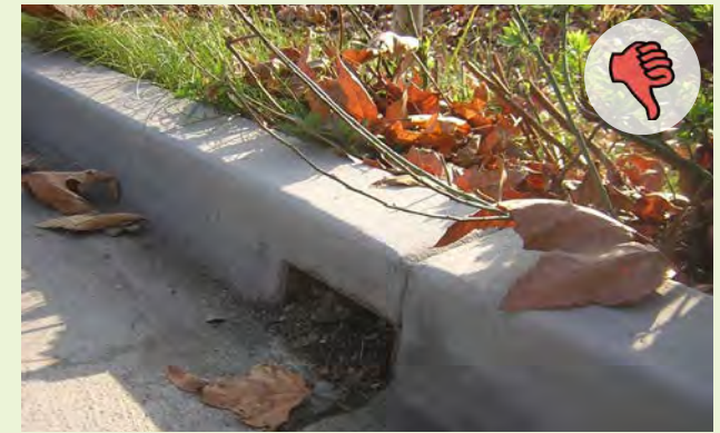
▲ A notched curb cut is way too small and constantly overloaded with sediment.
