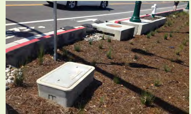
▲ Various utilities are elevated above the ponding elevation. Utility providers and contractors should be reminded that utilities should be located outside of green infrastructure areas if possible.
