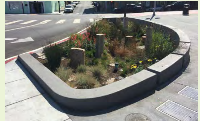
▲ This stormwater planter's edge is designed as a seat wall and includes gaps to allow runoff from the adjacent sidewalk to flow into the stormwater facility.
