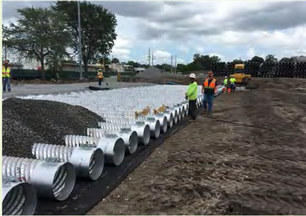
▲ A variety of systems and materials can be used to provide subsurface infiltration.
