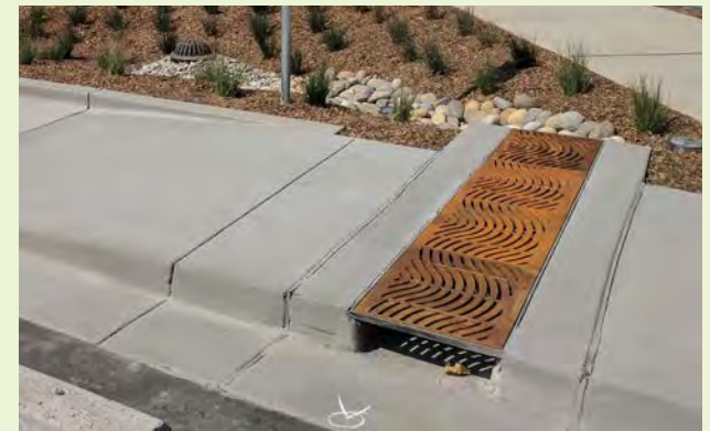
▲ Trench drains that are wider and straight are less likely to clog. Consider metal topped curb inlets at curbs where bus and truck loading areas and vehicle parking stalls are to limit damage to the trench drain grate and frame.
