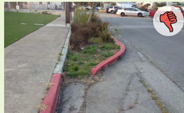
▲ This stormwater curb extension has no concrete forebay. Sediment builds up and blocks runoff from entering.
