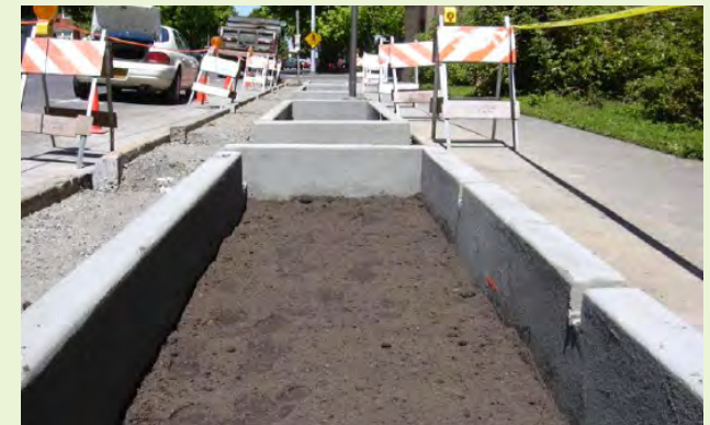
▲ New imported soil is placed within a planter. The imported soil's finish grade is set 3 inches lower to allow for a mulch layer.
