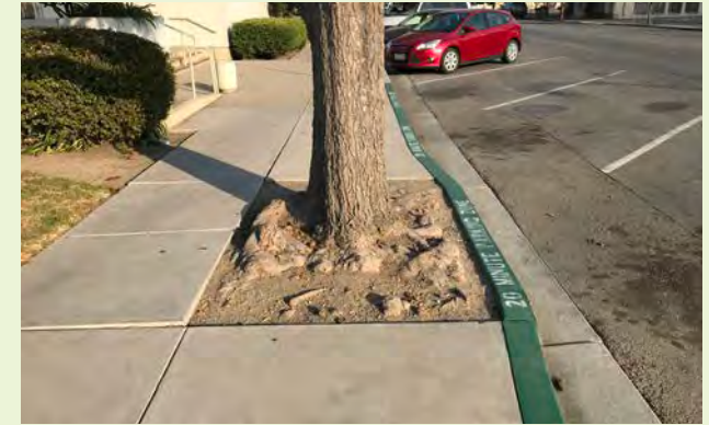
▲ This street tree unfortunately was not given enough room to grow between the street and sidewalk within a downtown environment.
