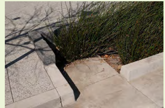
▲ This stormwater planter features a concrete sediment forebay that can be cleaned easily using a flat-bed shovel.
