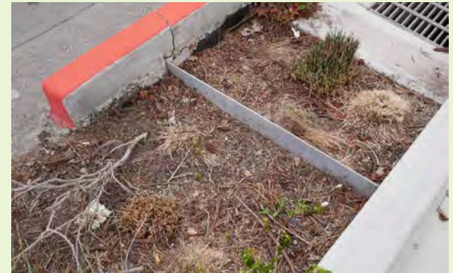
▲ Excessive plant trimming has caused severe plant dieback and eventual plant death.
