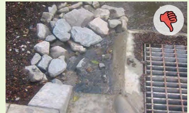
▲ A curb cut placed immediately adjacent to the overflow inlet does not allow runoff to enter the landscape and instead flows directly into the inlet.
