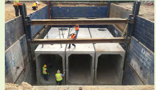
▲ After excavation of the project site, concrete chambers are lowered into place to store diverted stormwater below the park's open space.
