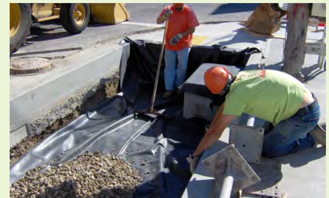
▲ A geotextile liner is installed within a flow-through stormwater curb extension to prevent infiltration near a utility vault.
