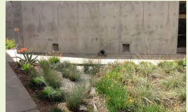
▲ This rain garden at the UC Davis campus captures roof runoff and features drought-tolerant plantings.
