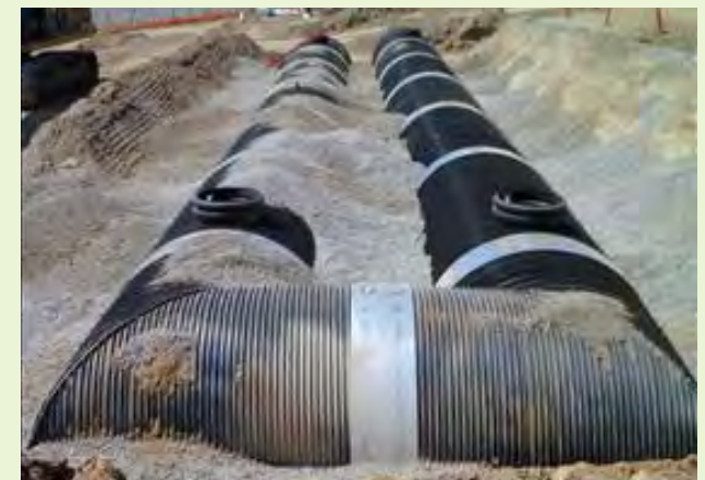
▲ Pretreatment of runoff is needed prior to the water entering the system.
