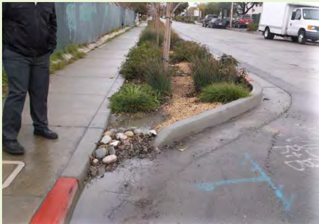
▲ River rock used to minimize erosion inhibits flow and creates sediment accumulation that is difficult to remove.
