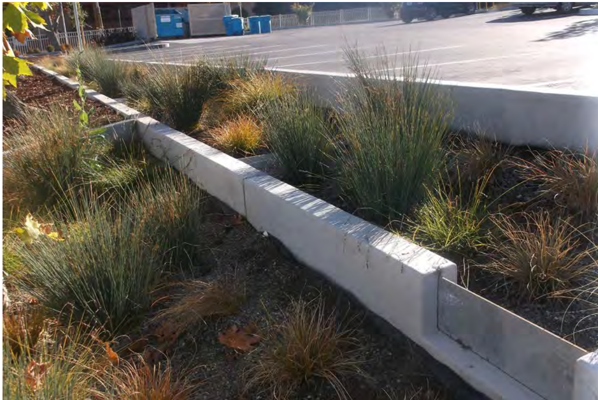
▲ This parking lot features a narrow infiltrative stormwater planter with a series of metal check dams that help slow and retain runoff.
