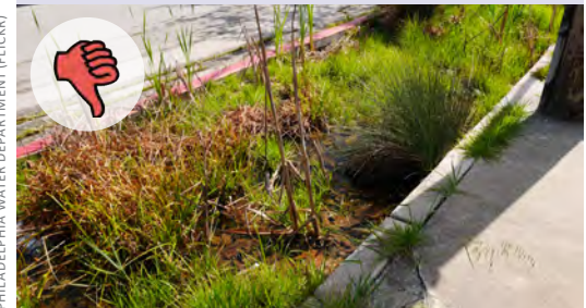
Poor, Overhaul Maintenance Routine
