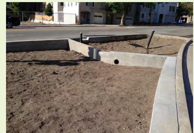
▲ Soils shall be stabilized for the placement of all structural elements including planter walls and adjacent pavements.
