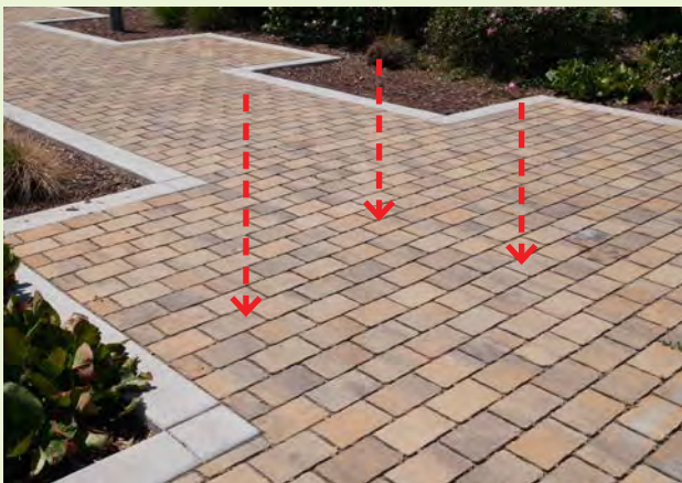
▲ This application of permeable pavers only has direct rainfall to manage. There is no impervious area runoff directed to it.
