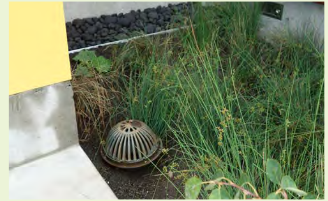
▲ Beehive drain in a building-adjacent stormwater planter.
