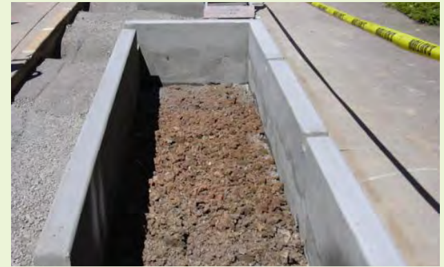
▲ During the construction process, the native soil is rototilled or broken up by other means to limit compaction.
