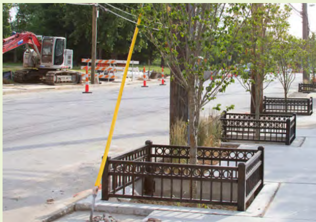
▲ Series of tree well filters along a retrofitted street.
