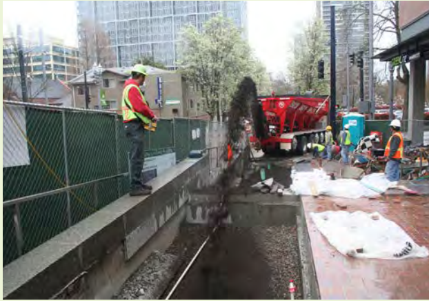
▲ Imported soil is being “delivered” to stormwater planters by means of a conveyor belt shooting the soil mix from 50 feet away. The entire process is orchestrated via remote control by the contractor and landscape architect.
