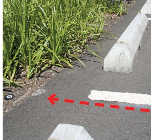
Figure 5-16: Stormwater runoff enters the stormwater facility through the 3-foot space between these wheelstops. The design could be improved by providing more drop in grade between the asphalt and landscape area. (Credit: SMCWPPP, 2009)
