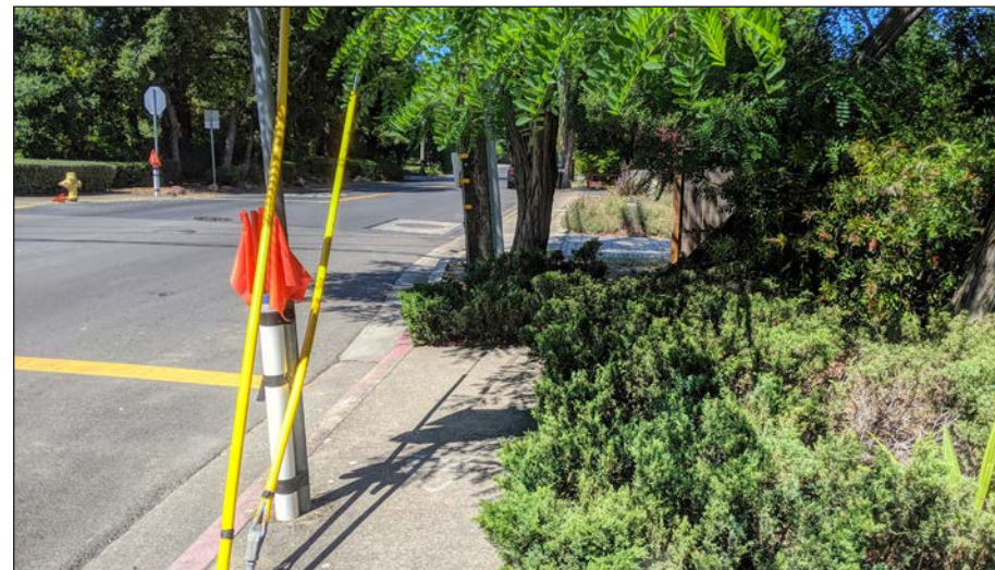
The sidewalk on the south side of Sharon Road at Altschul Avenue is interrupted by landscaping, and the crossing lacks a curb ramp.
