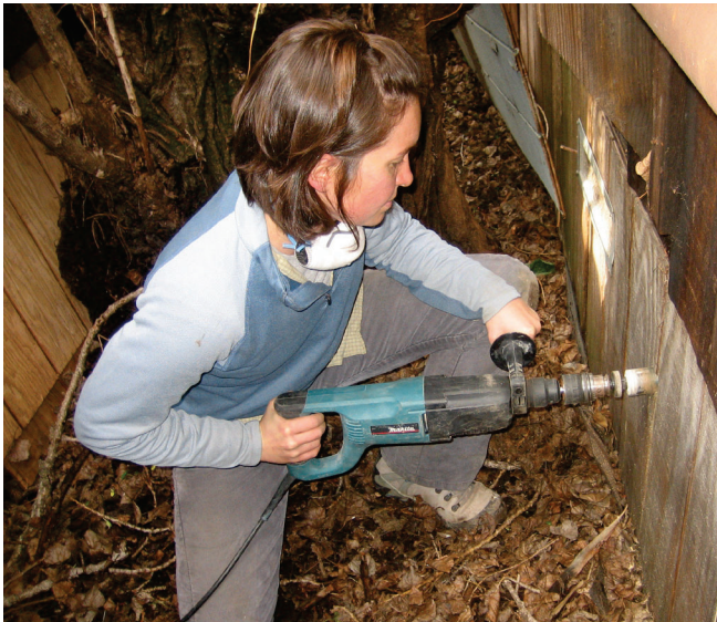
Drilling a 1½-inch hole for pipe. Note: A pilot hole was drilled first. Photo: Laura Allen.
