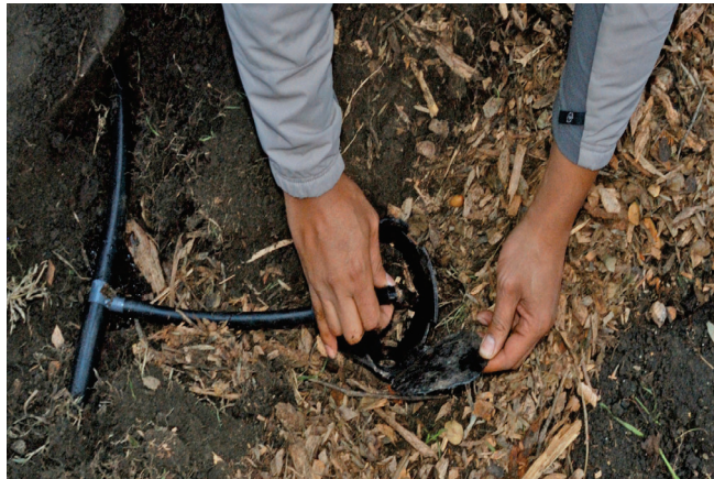
Adjusting flow by rotating the tees. Ball valves can be added to the ends of small tubes, if necessary. Photo: David Glover.
