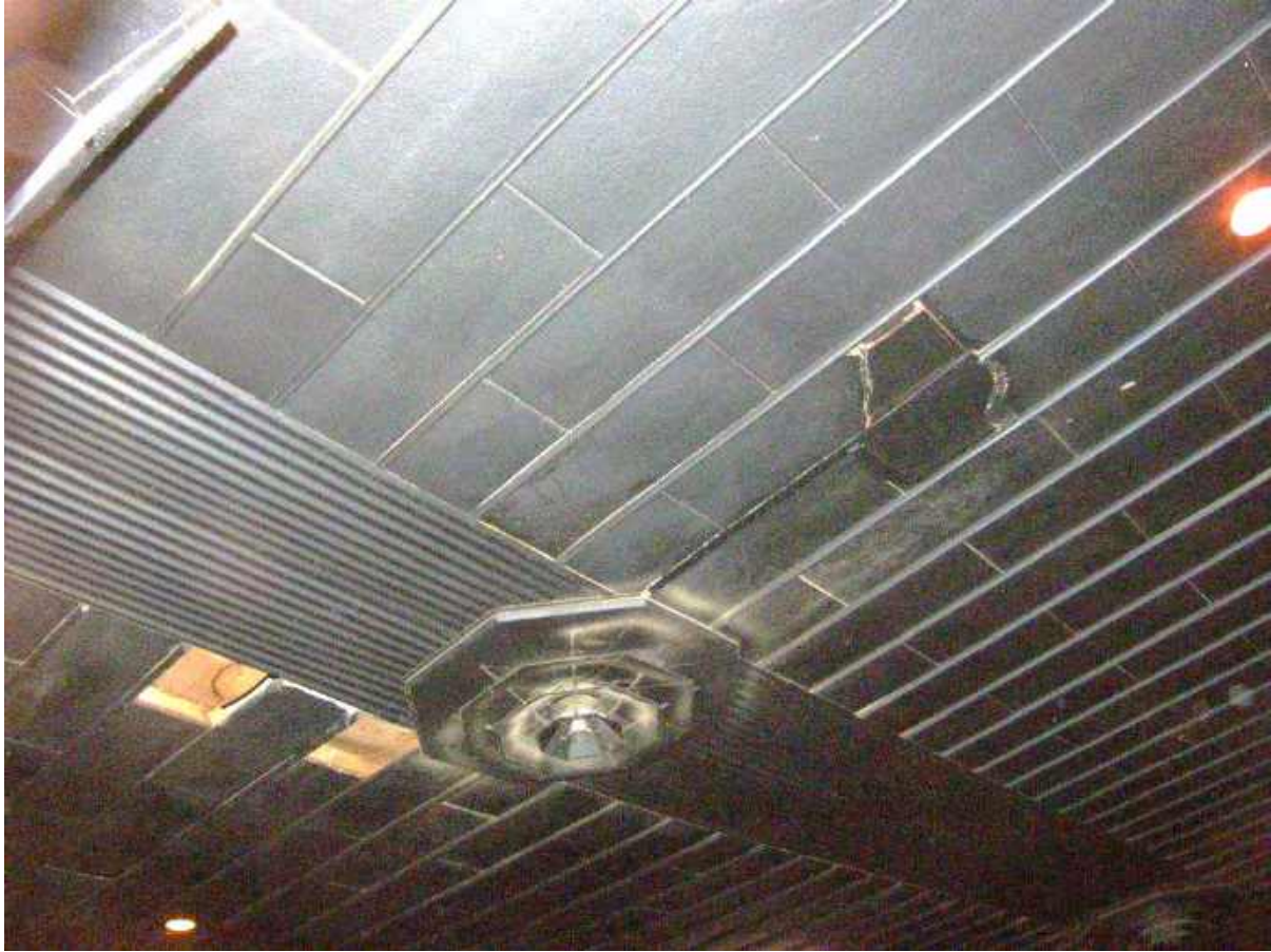
Photograph 7 – 949 El Camino Real- Guild Theater View: Interior of the auditorium showing the ceiling of celotex and panels,
