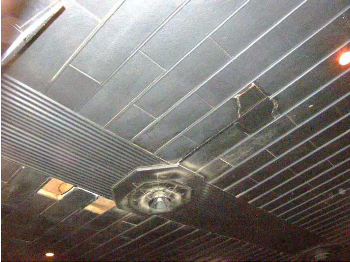
Photograph 7 – 949 El Camino Real- Guild Theater View: Interior of the auditorium showing the ceiling of celotex and panels,
