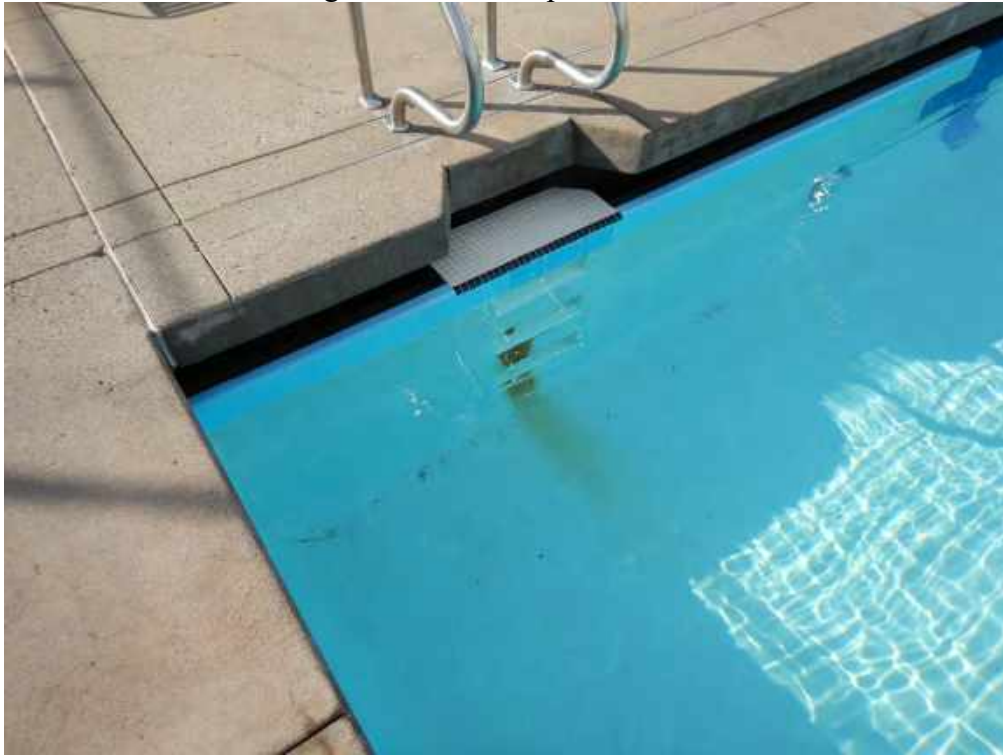
Photos 18 and 19 Staining from rebar “seep” on two sets of built-in ladder stairs
