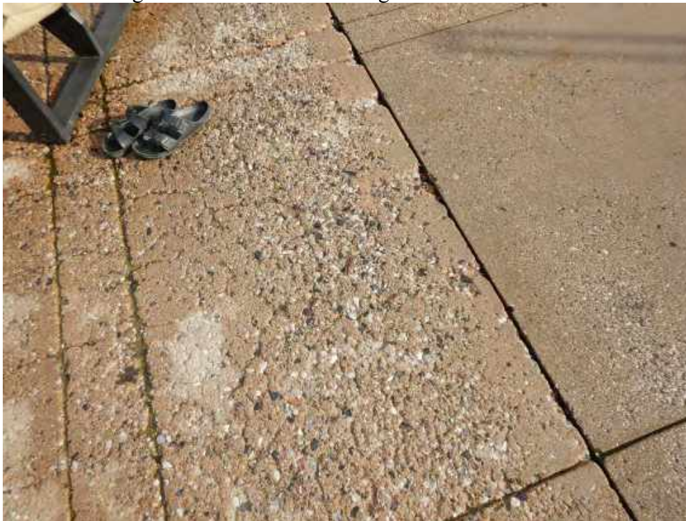
Photos 5 through 10 – Pool Deck Surfacing Condition
