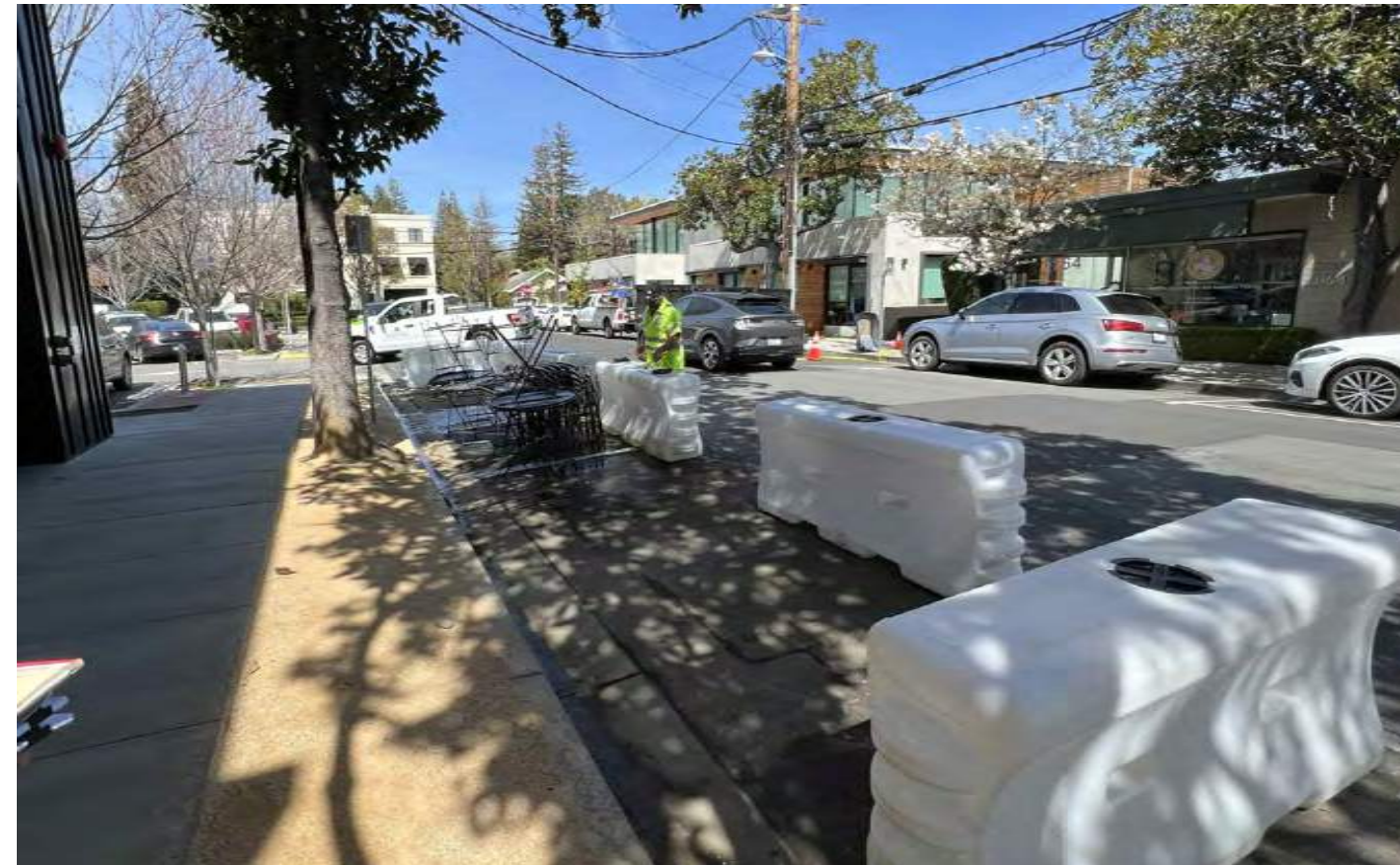
Photo of non-compliant items 1 through 5.
