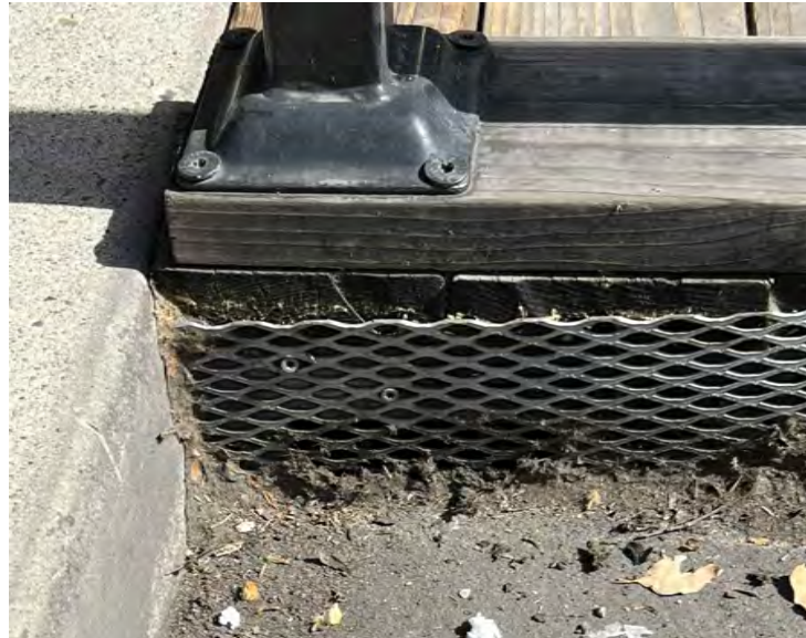
Photo of non-compliant item 3.
