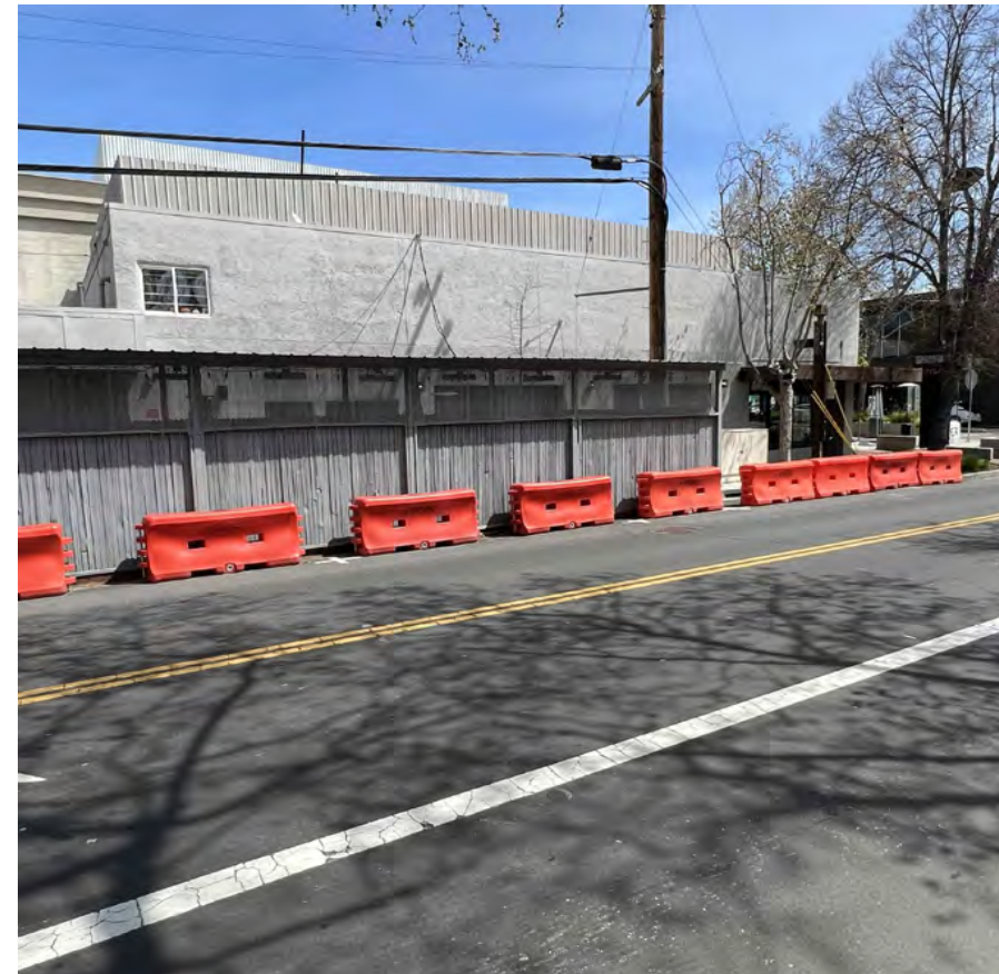
Photo of non-compliant items 1, 2, 3 & 7.
