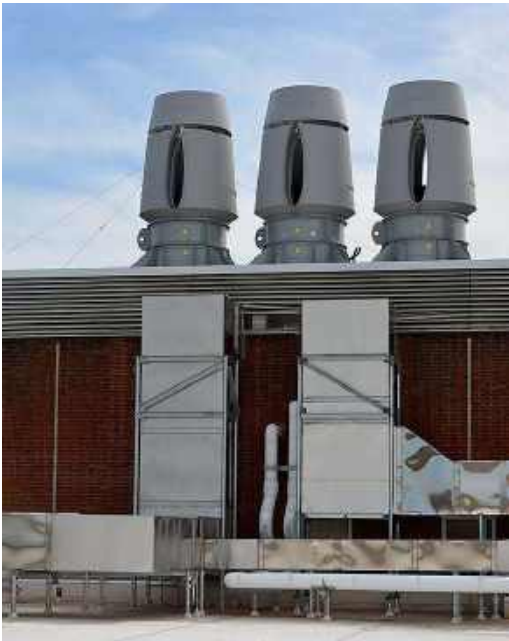
Figure 1 – Biolab Exhaust Stacks
