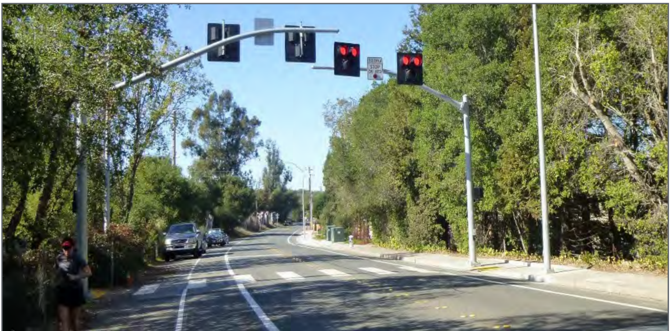
Crossing signals such as this one, called a pedestrian hybrid or HAWK beacon, can help drivers become more aware of people walking.
