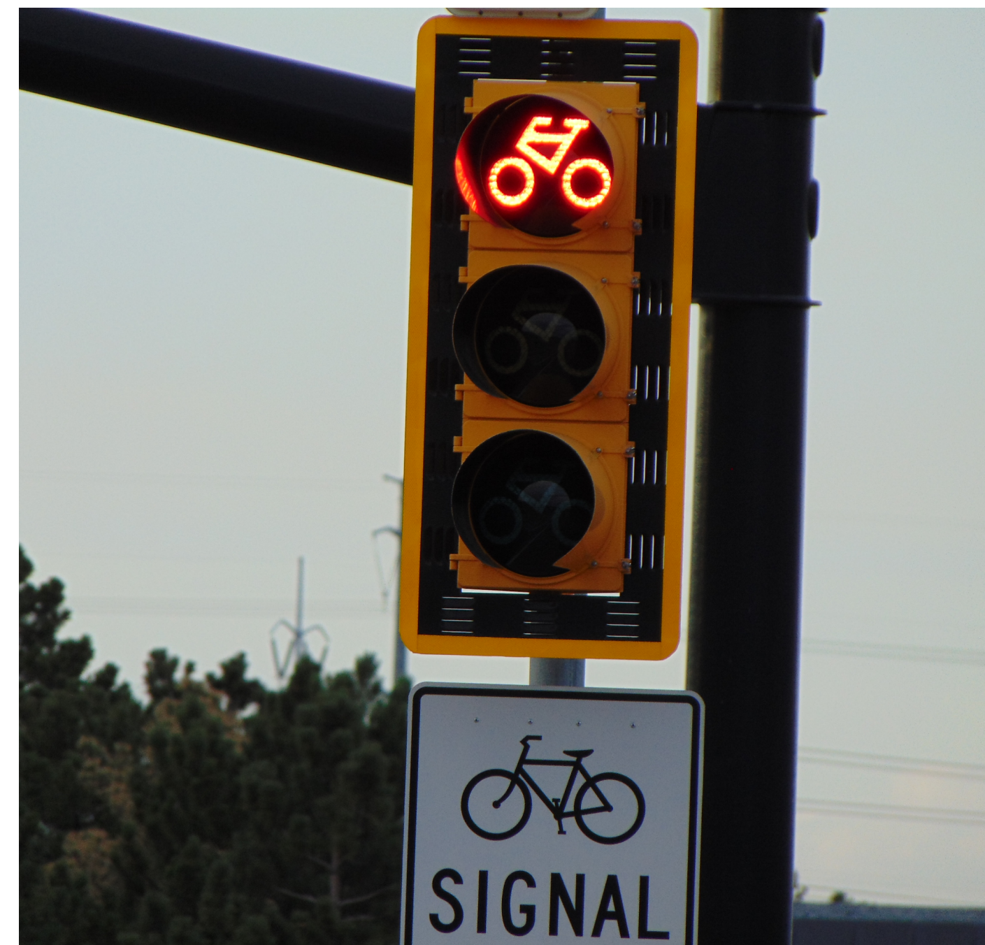
Bicycle Signal Provides separate signal phase for bicyclists, reducing conflicts with vehicle movements
