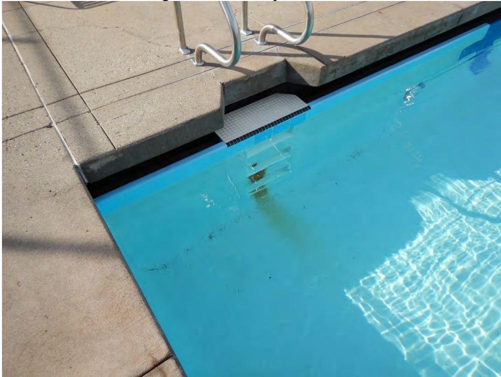
Photos 18 and 19 Staining from rebar “seep” on two sets of built-in ladder stairs
