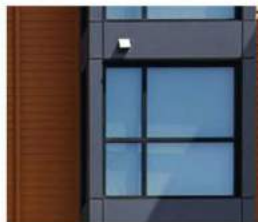
W1 VINYL WINDOW VPI QUALITY WINDOWS BLACK FRAME FINISH OR SIMILAR BY ALTERNATIVE MANUFACTURER
