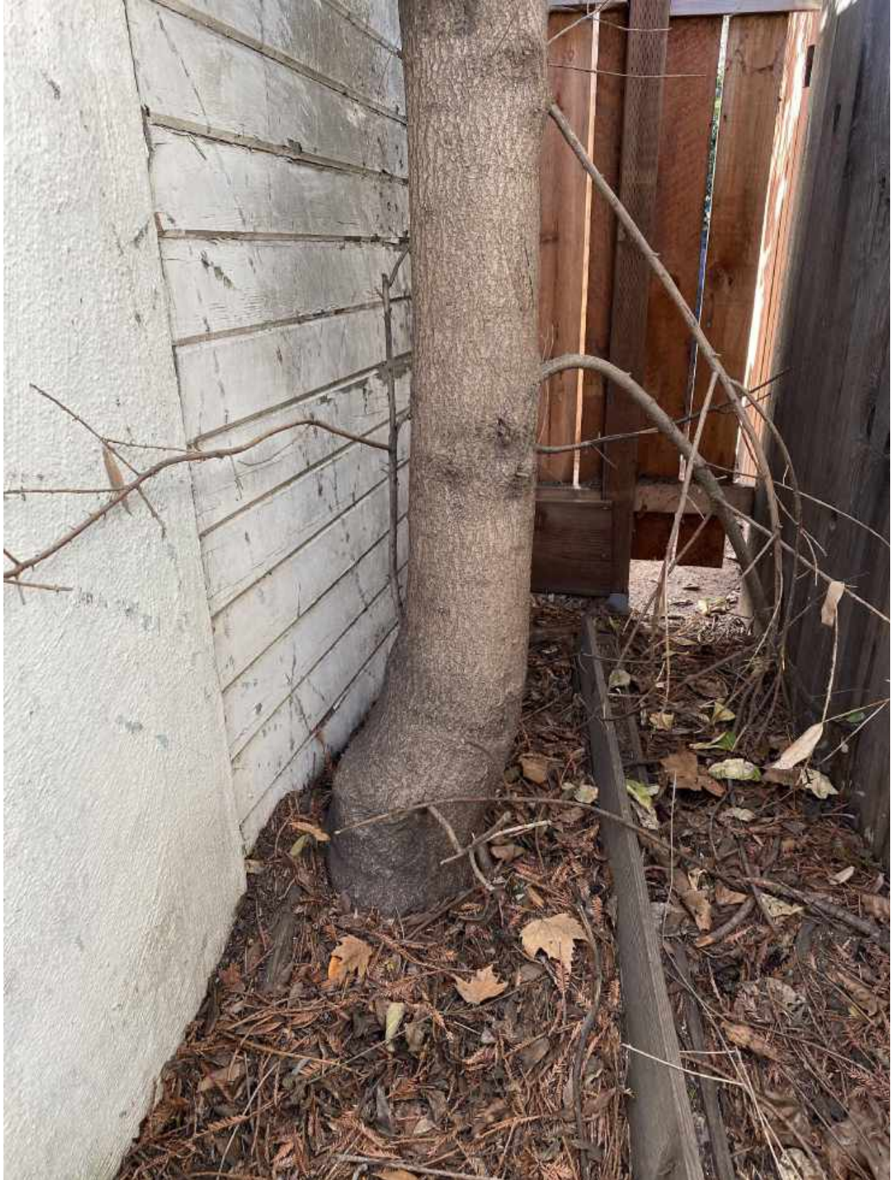
Photo 5. Closer view of the proximity of the trunk of tree #3 to the existing detached garage.
