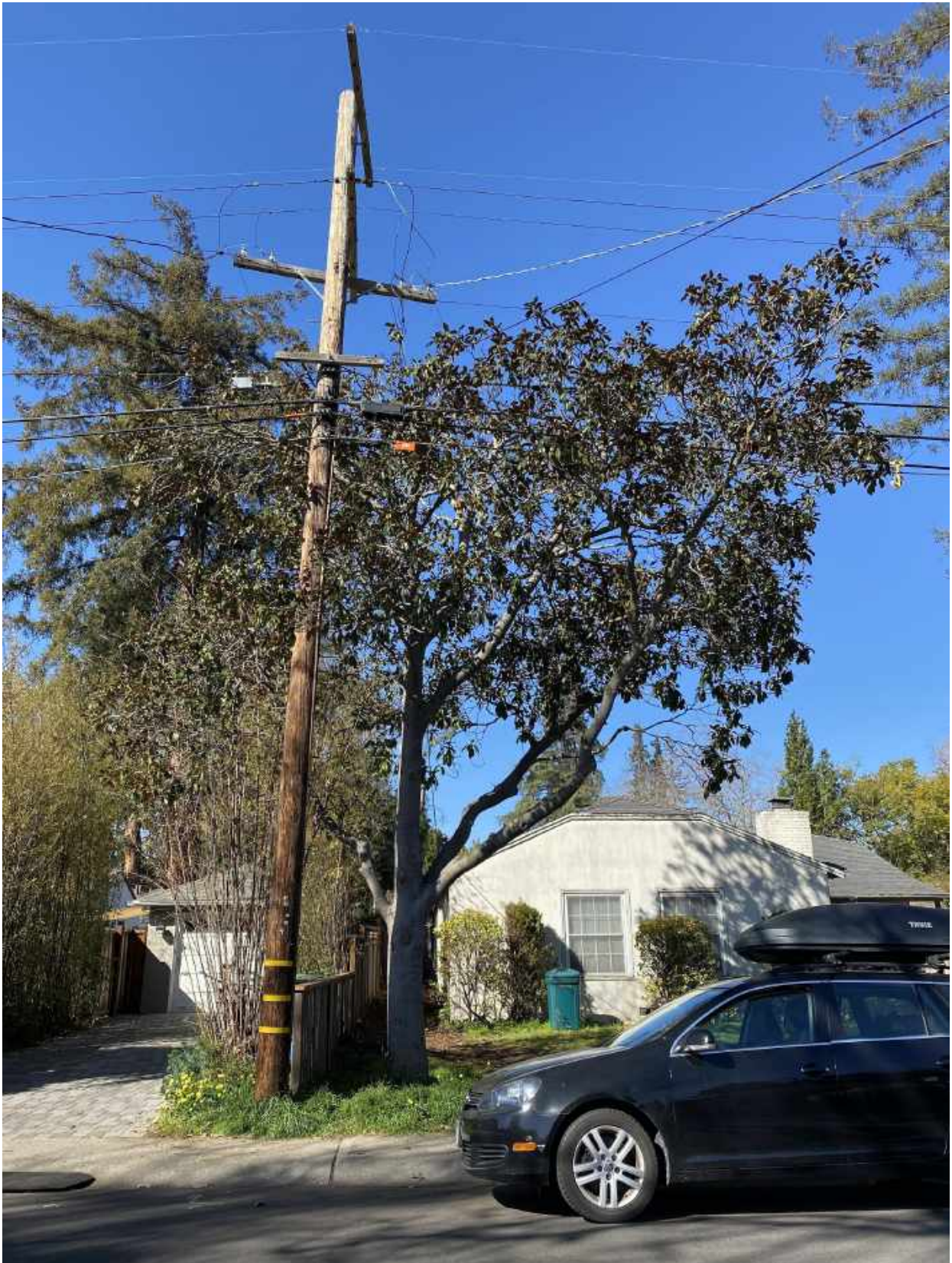
Photo 11. View of tree #2 from McKendry Dr. This species of tree is unsuitable under utility lines and was showing signs of stress. Construction impacts may be moderate to severe.
