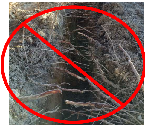
Figure 8: How not to trench
